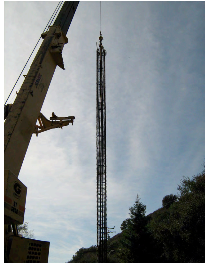
A crane moves a re-bar support column into place during construction activities.
