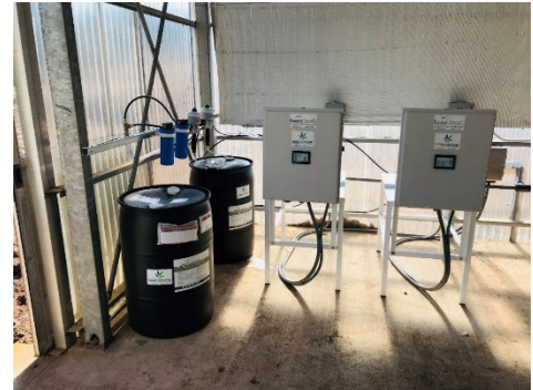
Odor Pumping equipment
