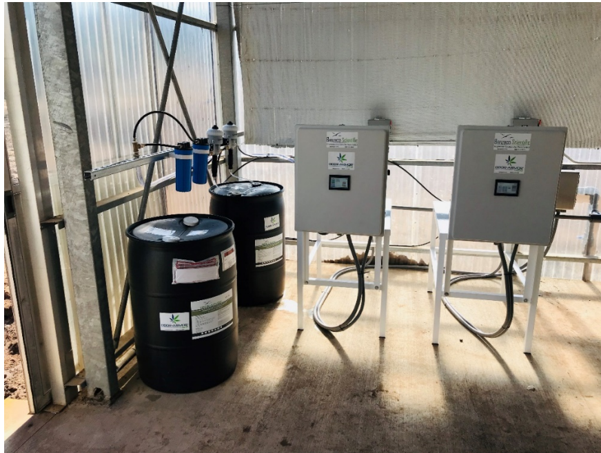
Odor control pumping systems at Valley Crest Farms
