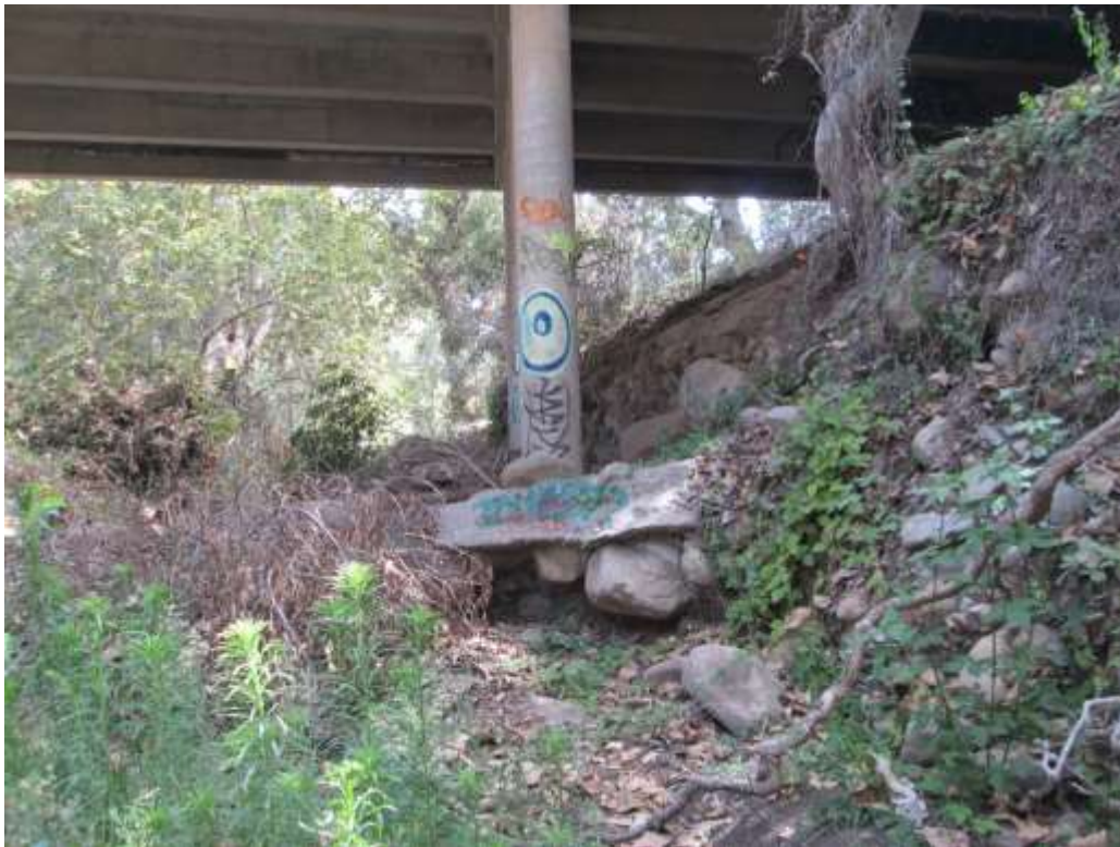
Existing Scour Protection Padaro Lane Br. No. 51C-0163 over Toro Canyon, looking south
