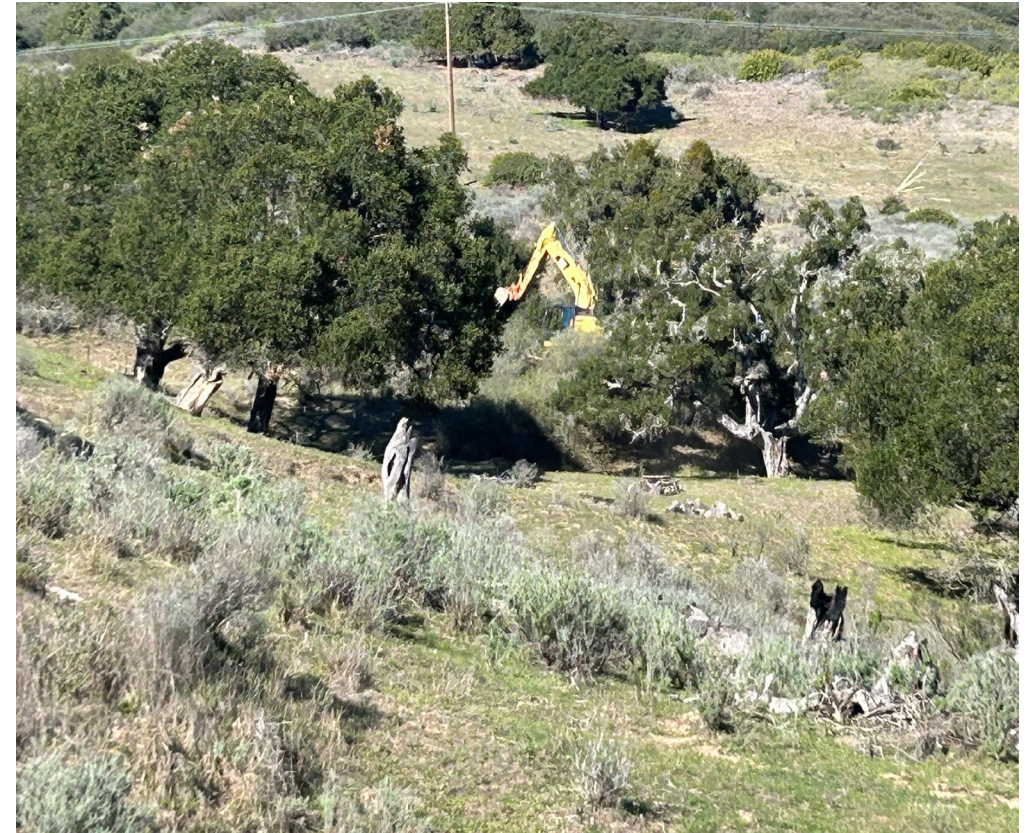
Unpermitted Repair Work; Ignoring Cease and Desist
