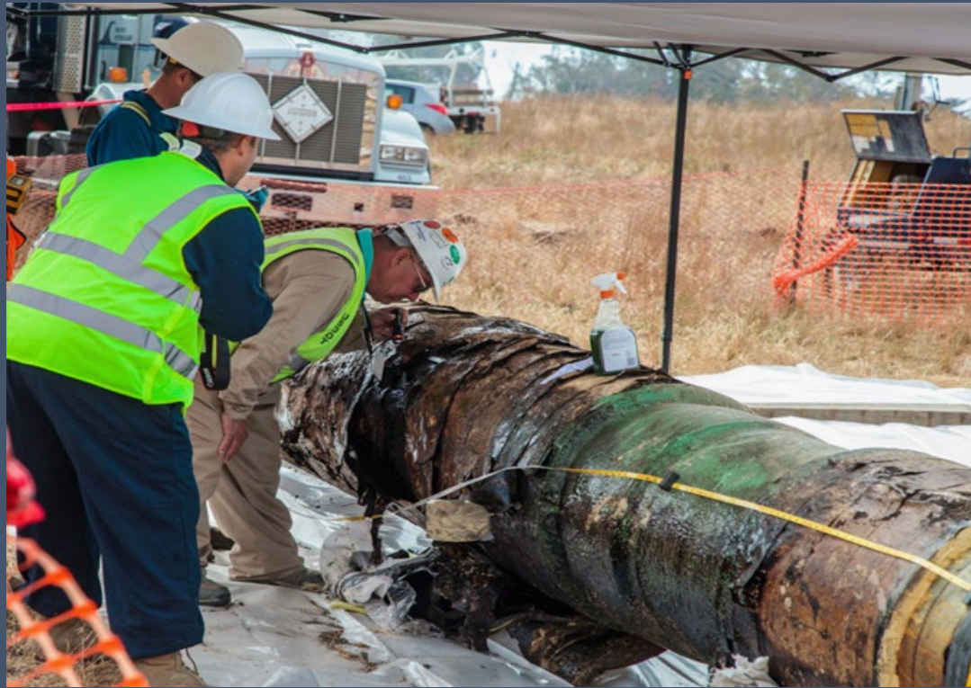
Sable's Defective Pipeline Credit: Bill Reitherman
