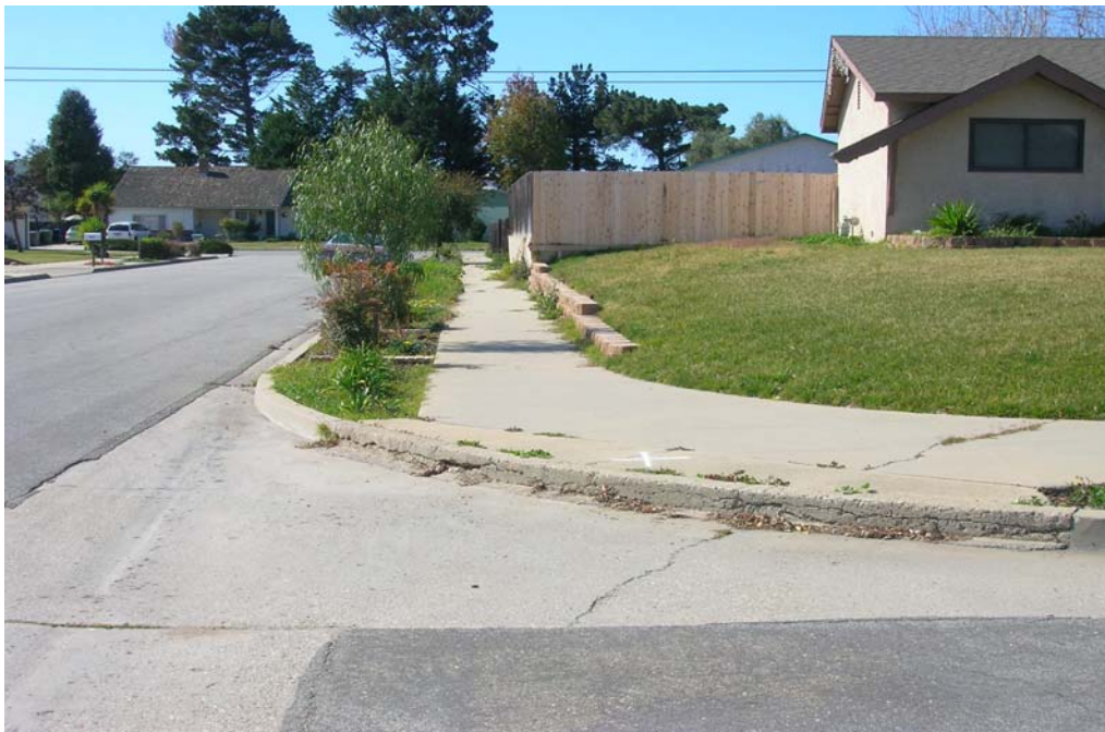
Typical site for concrete repairs; at this site the spandrel will be repaired and a new ADA-compliant curb ramp will be constructed.
