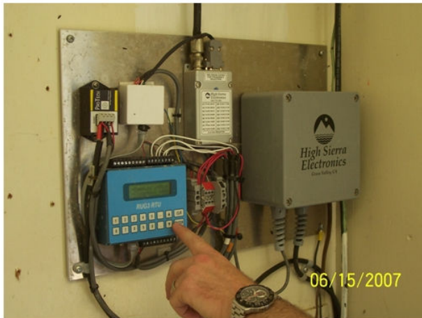
Water Level & Gate Opening ALERT Gauging (RUG3)
