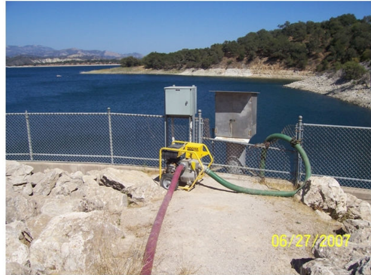
Cachuma Reservoir / Water Level Gauge (Shaft Encoder)
