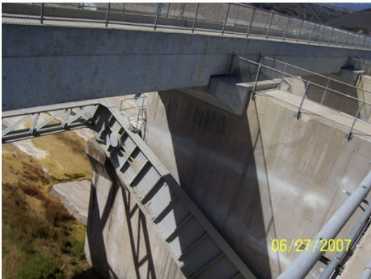
Dam Gates & Inclinometers
