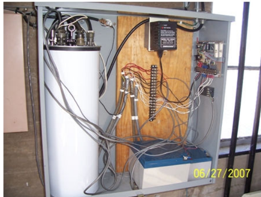
Reservoir Level & Gate Opening ALERT Instrumentation
