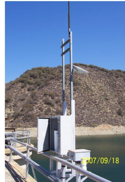
Water Level ALERT Instrumentation (Press. Trans.)
