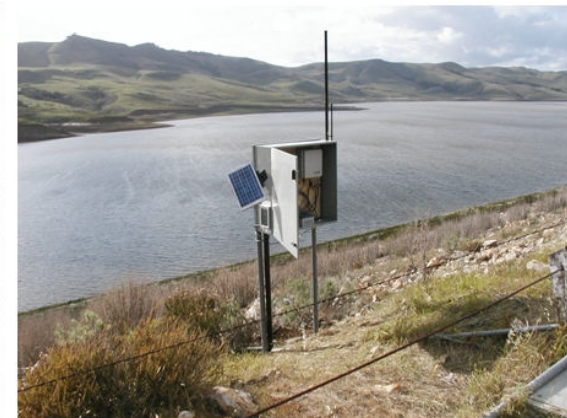
Reservoir & Level Instrumentation (Bubbler)
