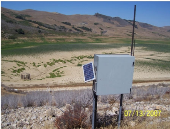
Reservoir Level Gauge Enclosure
