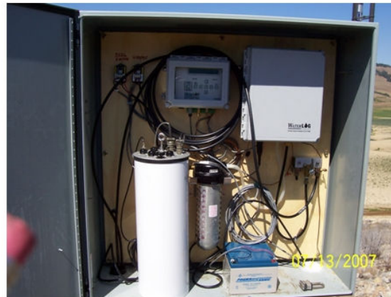
Reservoir Level Instrumentation (Bubbler)
