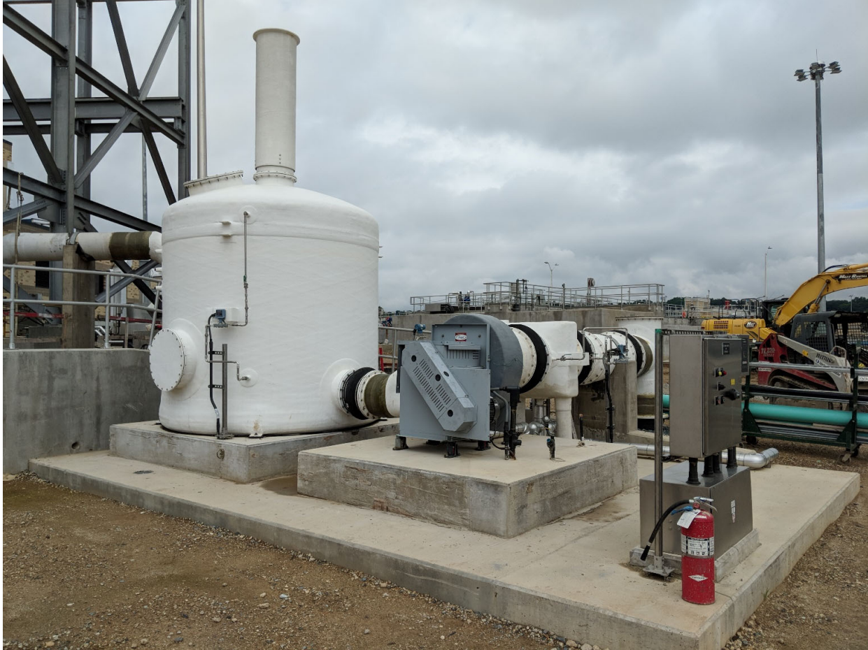
Figure 5.21 DCWater Carbon Adsorber Odor Control System
