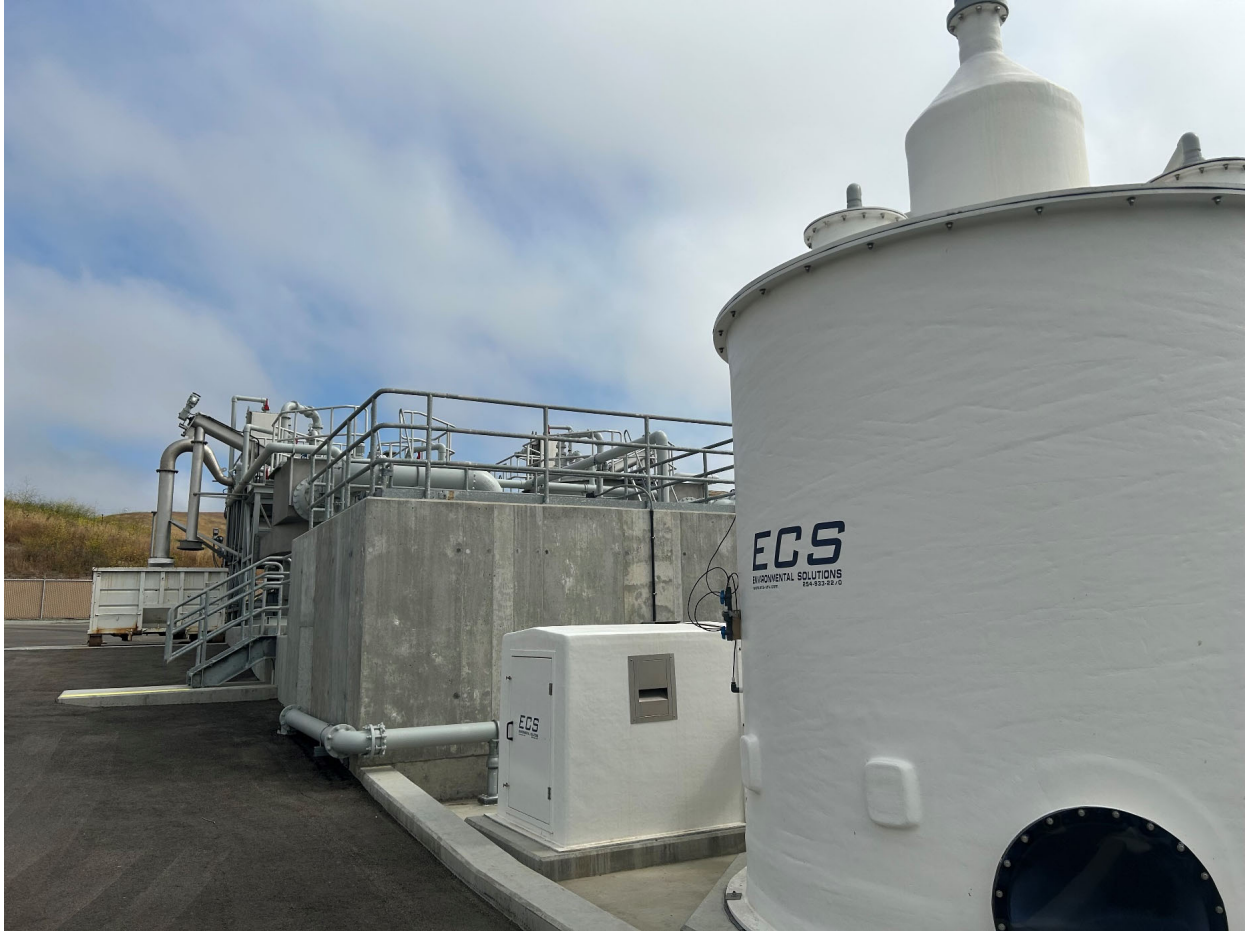
Figure 5.20 City of Morro Bay Screenings, Dewatering, and Odor Control System
