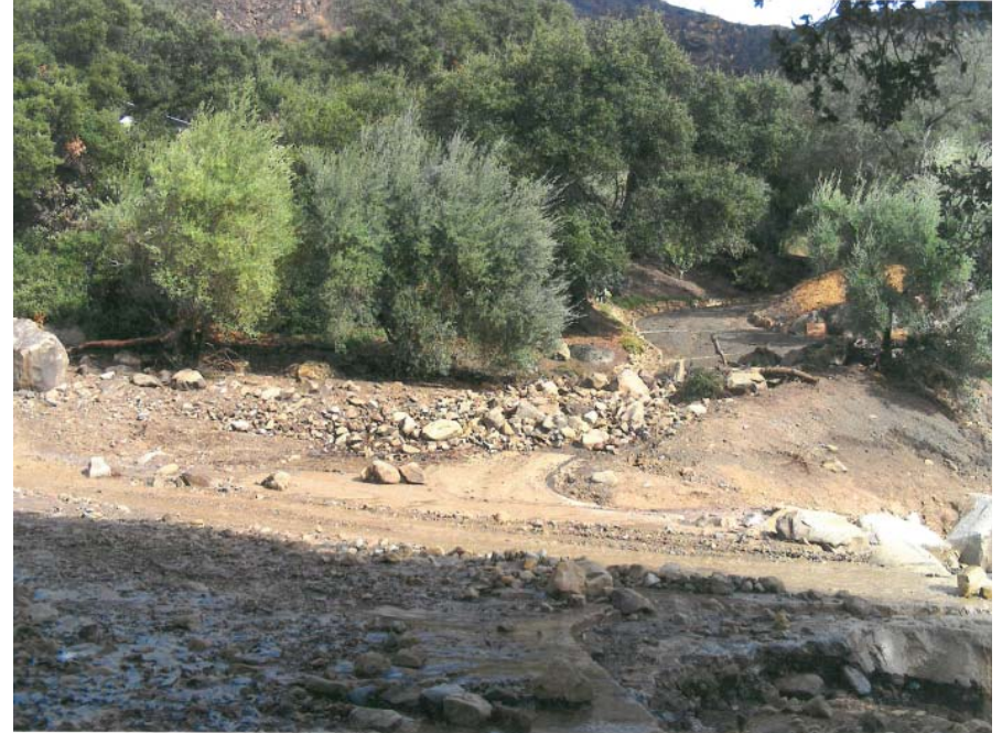
Easement road blockage view east. 1/9/18.
