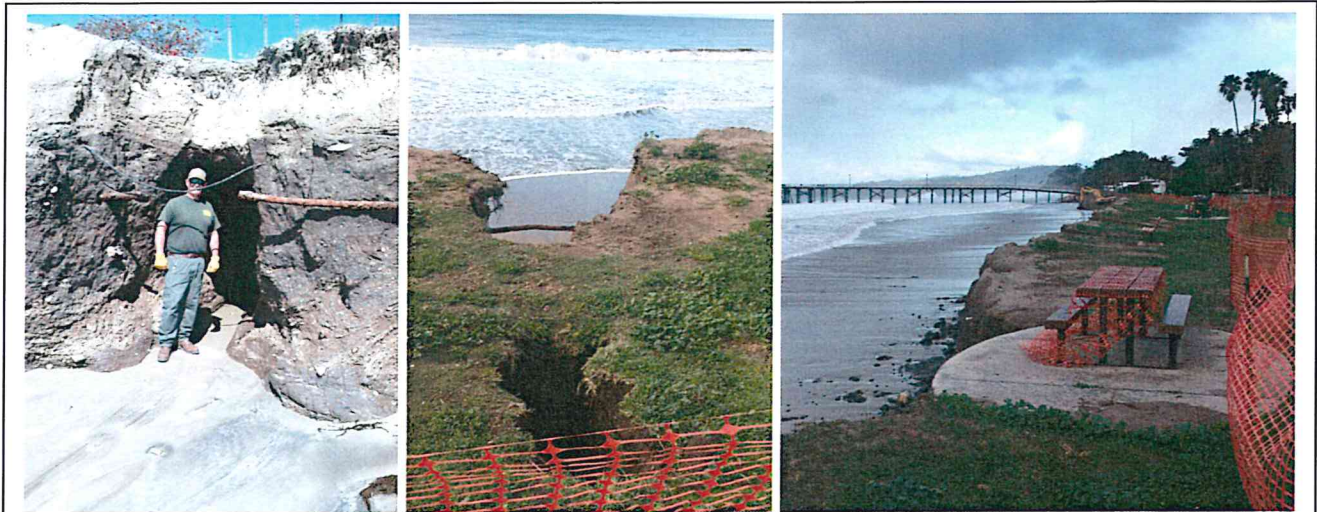
Sink holes that developed in March 2016 exceeded more than 10 feet in depth in some locations (left), with crevasses extended 15-20 feet deep into the lawn resulting in imminent substantial impacts to public safety at the park. The County took permitted emergency action to cordon off and fill these areas and to initiate repairs.
