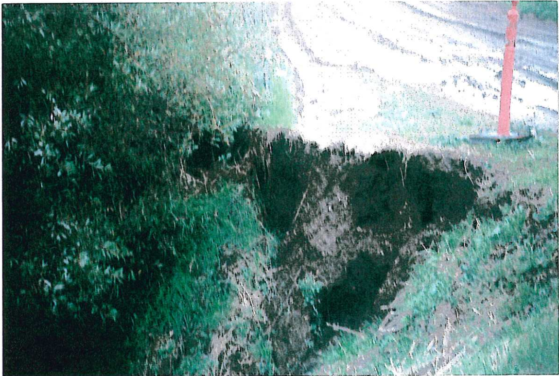
Damage and threat to life
