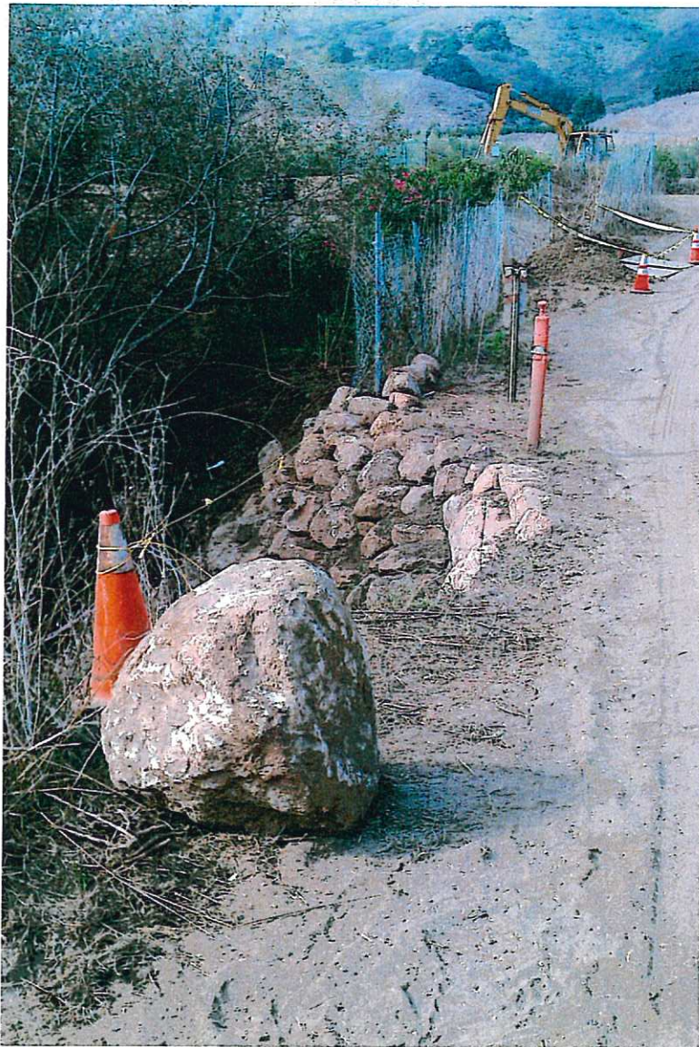
Lining of damage called a repair.
