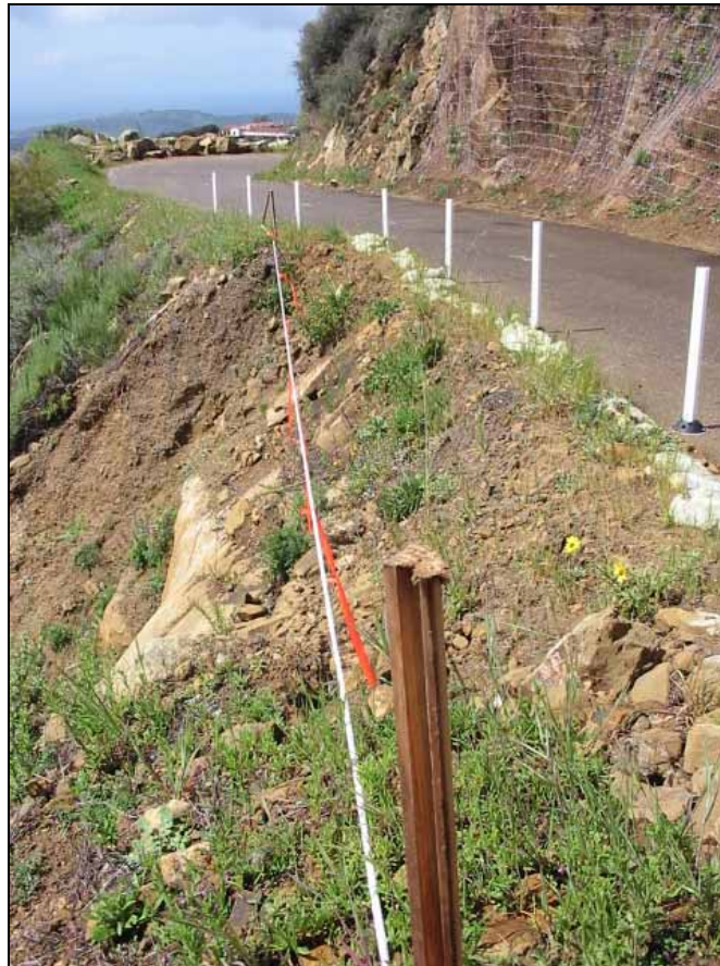
Photo: Existing site condition, with white tape line approximating extent of lost shoulder width (Looking South)
