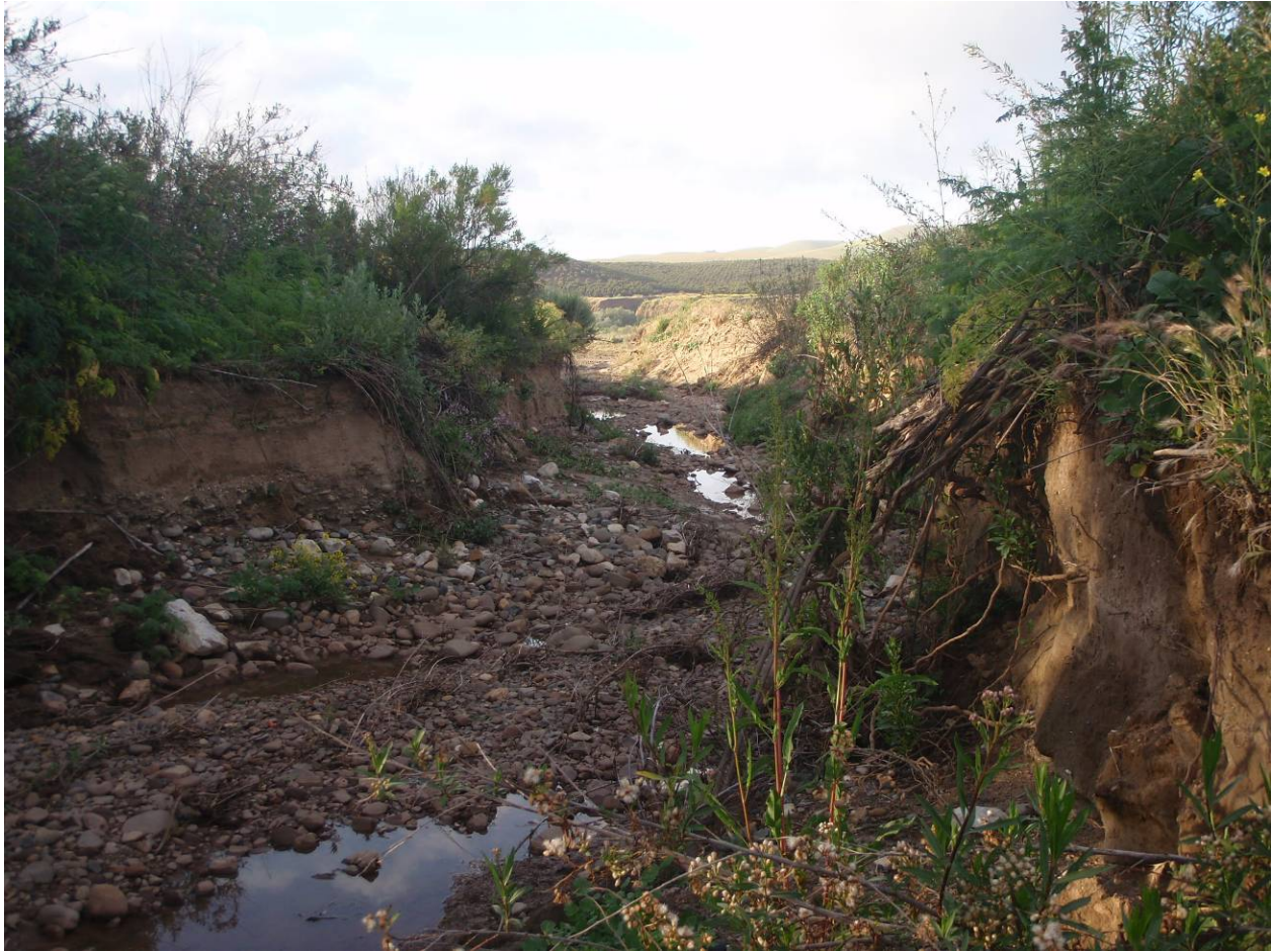
Figure 6: Outflow of culvert pool showing steeply downcut banks.
