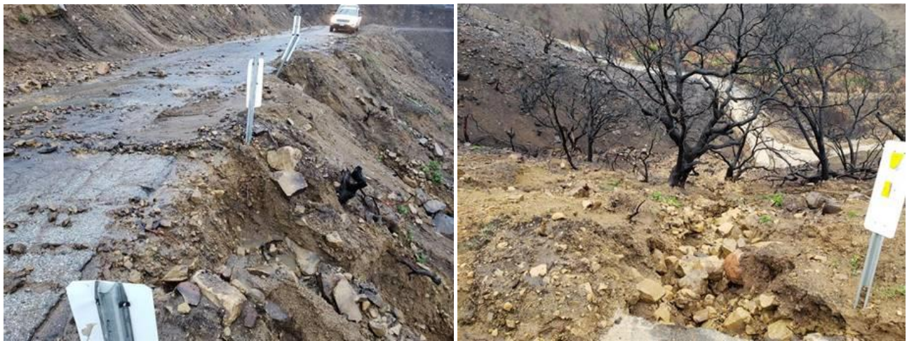
Alisal Fire, Refugio Road MP 4.0
