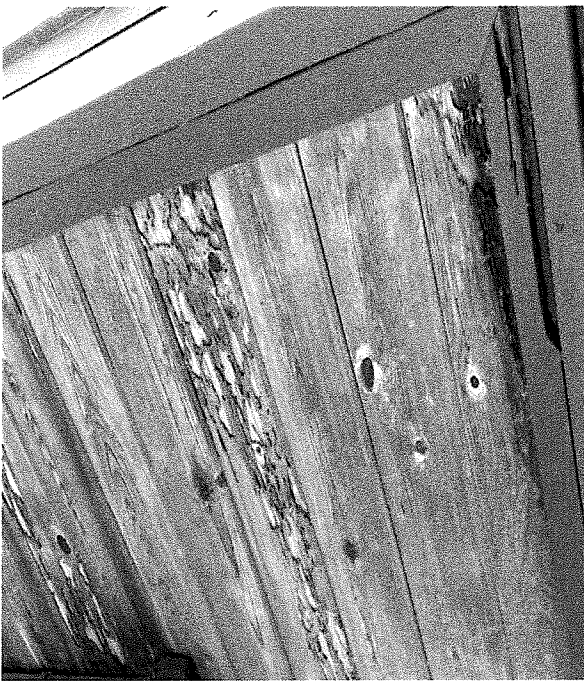
Termite damage and wood rot (Bldg. 1)
