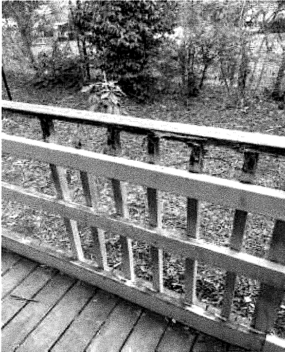
Rotted handrail outside Bldg. 2
