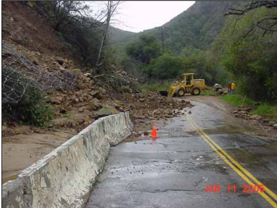
Stagecoach Road, with existing netting showing contained materials and adjacent, unprotected area where rock debris entered the roadway.
