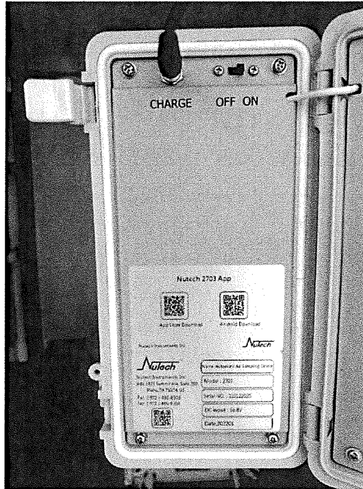
Figure 7: The Nutech 2703 controller is connected to a power source and is turned ON.
