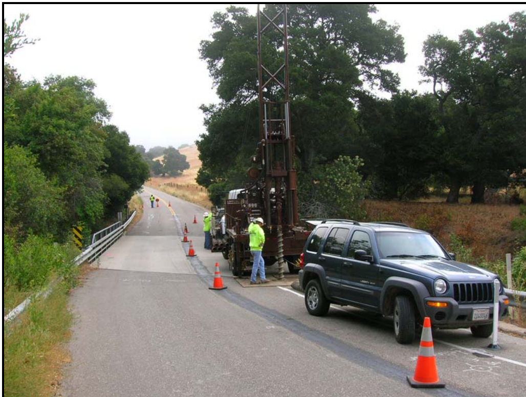
Preliminary Subsurface Geotechnical Investigation at Jalama Rd. Bridge (Looking east towards Highway 1)
