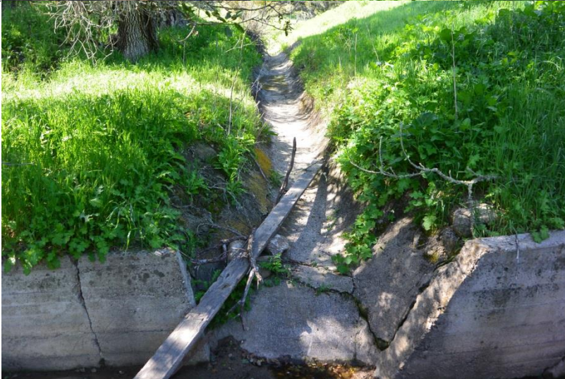
Photo 30. Concrete ditch (Class IV watercourse) that conveys water into man-made drainage system (Class IV watercourse). (photo taken 3/26/2019)
