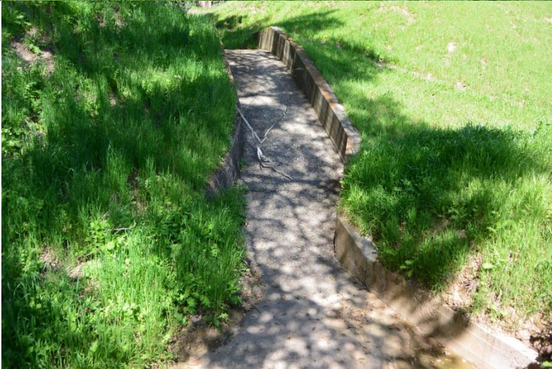
Photo 32. Concrete ditch (Class IV watercourse) that conveys water into man-made drainage system (Class IV watercourse). (photo taken 3/26/2019)
