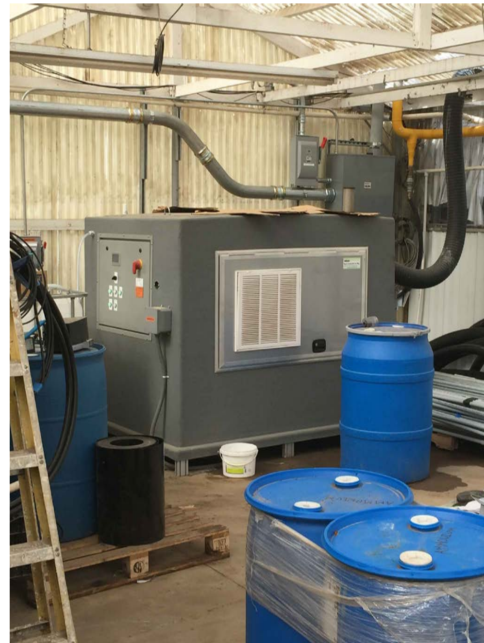
ODOR CONTROL UNIT
