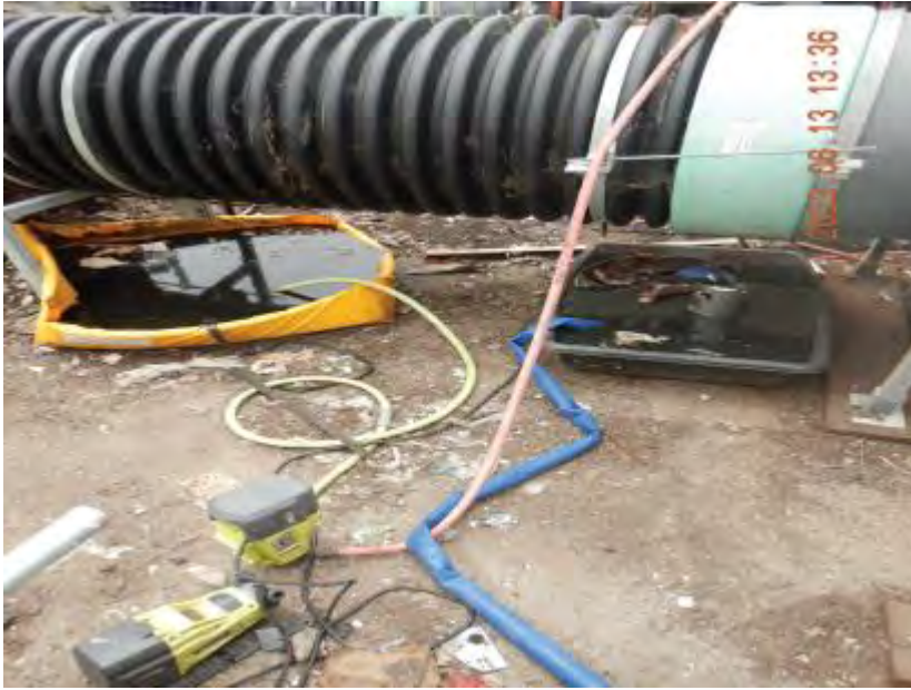
Photograph 28A. June 13, 2023. Collected wastewater beneath damaged pipe. Wastewater overflowing from bins.
