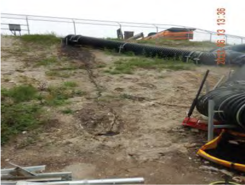
Photograph 27A. June 13, 2023. Wastewater flowing from damaged pipe onto landfill surface.
