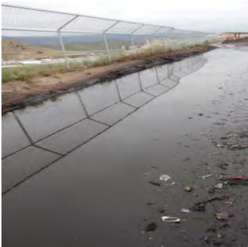
Photograph 12A. June 13, 2023. Pondered wastewater at the northern portion of the facility.
