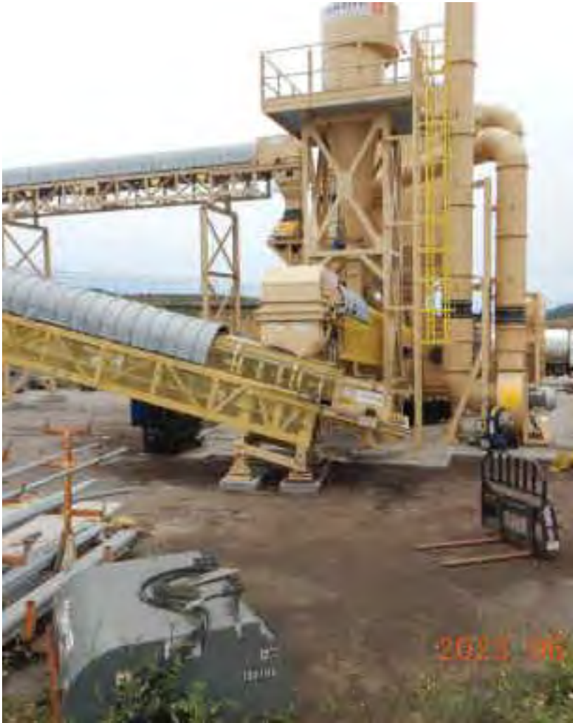
Photograph 2A. June 13, 2023. Compost on D-table working surface. No berm around this area of the CMU, as was included in the approved technical report for the site.
