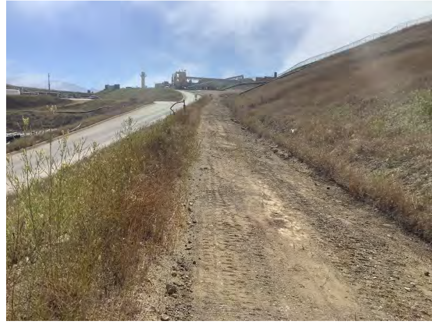
Photograph 36B. July 11, 2023. Stained soil has been removed and stored in a roll off bin.
