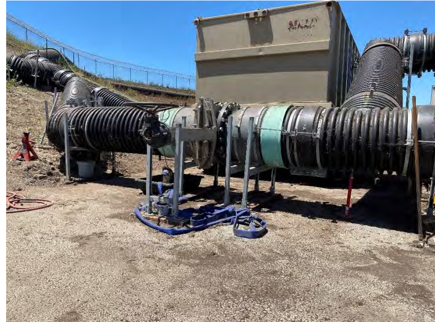
Photograph 28B. July 14, 2023. There is no longer collected wastewater below the conveyance system.
