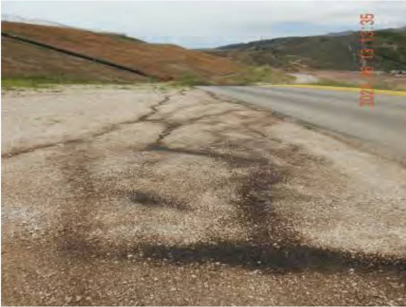
Photograph 26A. June 13, 2023. Wastewater flowing outside of the compost facility towards a lower landfill bench.
