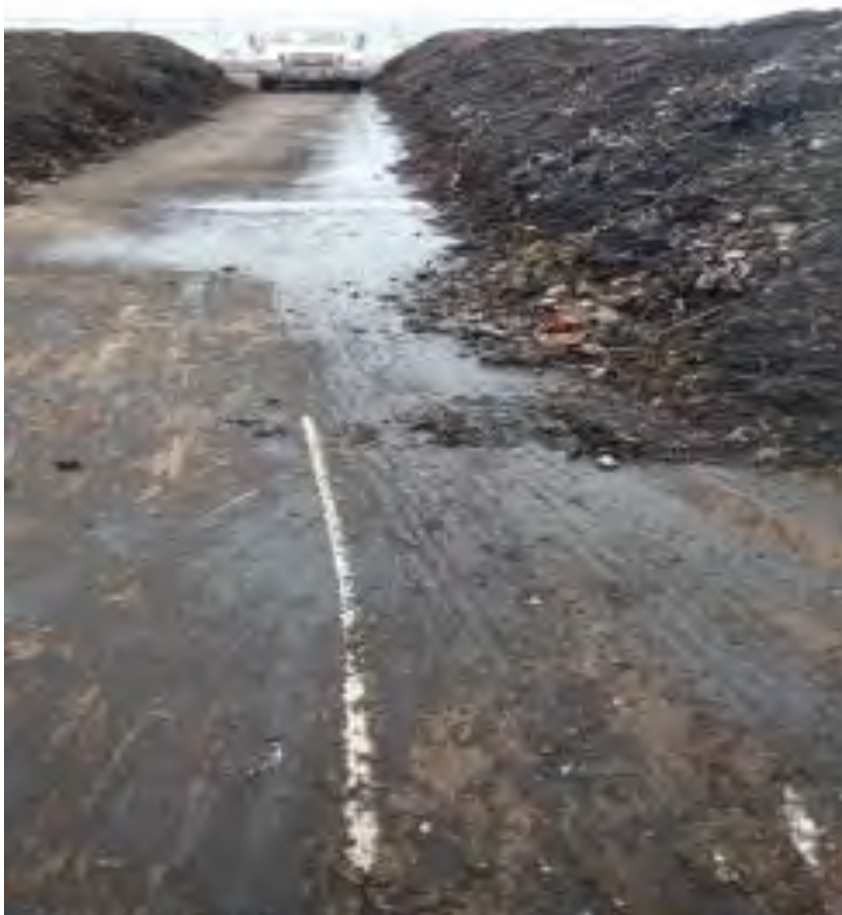
Photograph 11A. June 13, 2023. Damaged area of the working surface with ponded water and scraped asphalt surface.
