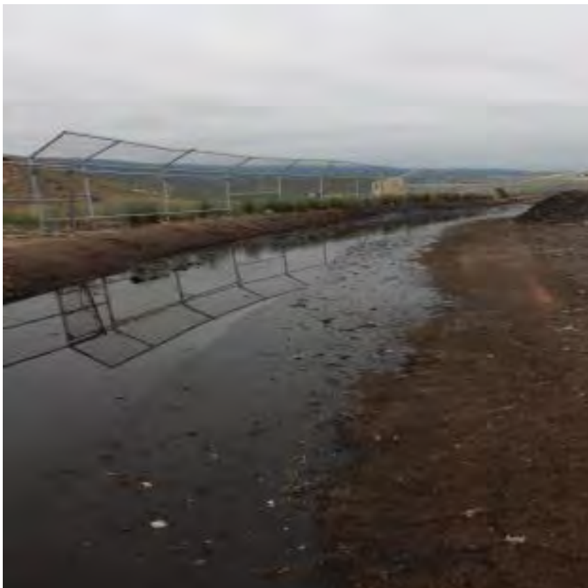
Photograph 8A. June 13, 2023. Pondered wastewater at the northern portion of the working surface.
