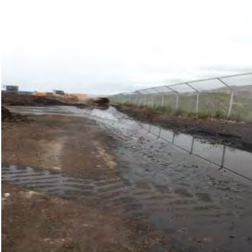
Photograph 9A. June 13, 2023. Pondered wastewater at the northern portion of the working surface with a scraper pushing compost/material into the ponded area after scraper dragged its blade around the perimeter of the working surface.
