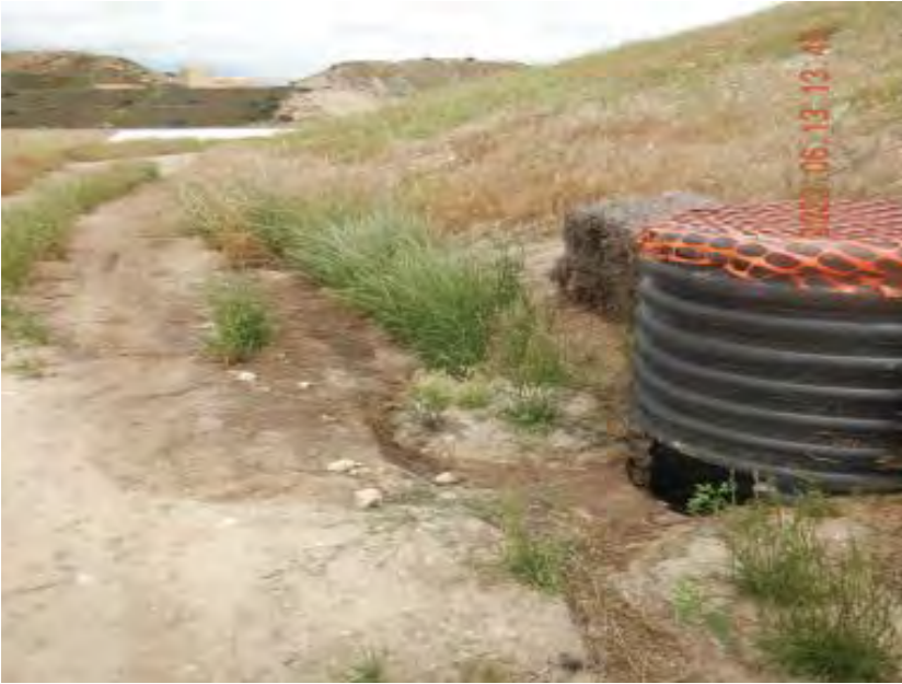
Photograph 34A. June 13, 2023. Wastewater flowing from the compost facility onto a landfill bench where it enters a second stormwater pipe connected to the south sediment basin.
