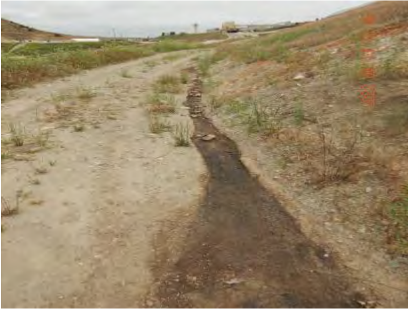
Photograph 36A. June 13, 2023. Wastewater flowing along landfill bench over an unlined area of the landfill.
