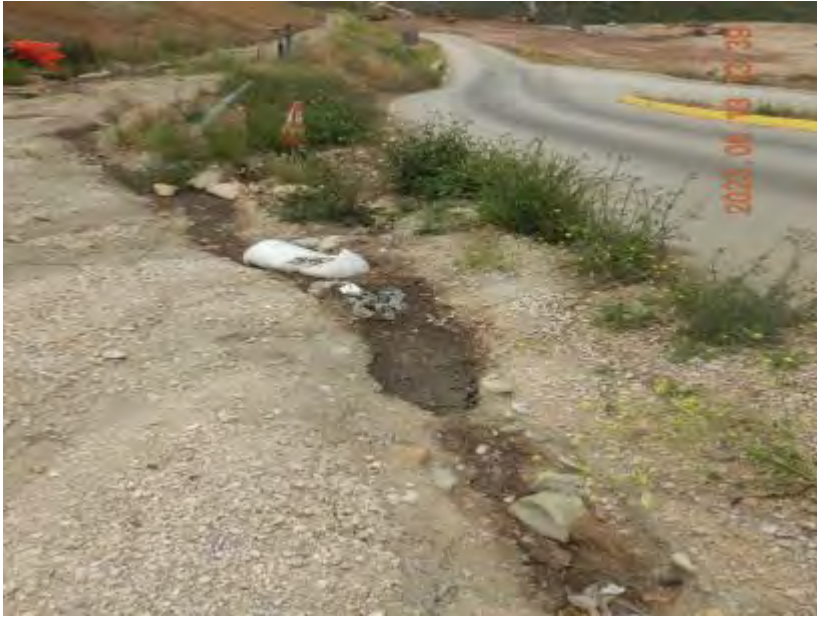
Photograph 31A. June 13, 2023. Wastewater flowing from the D-table area towards a lower landfill bench.
