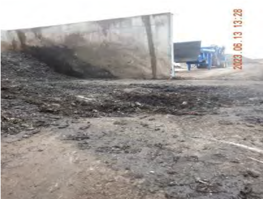
Photograph 22A. June 13, 2023. Damaged working surface where feedstock/digestate enters the facility from the ADF.
