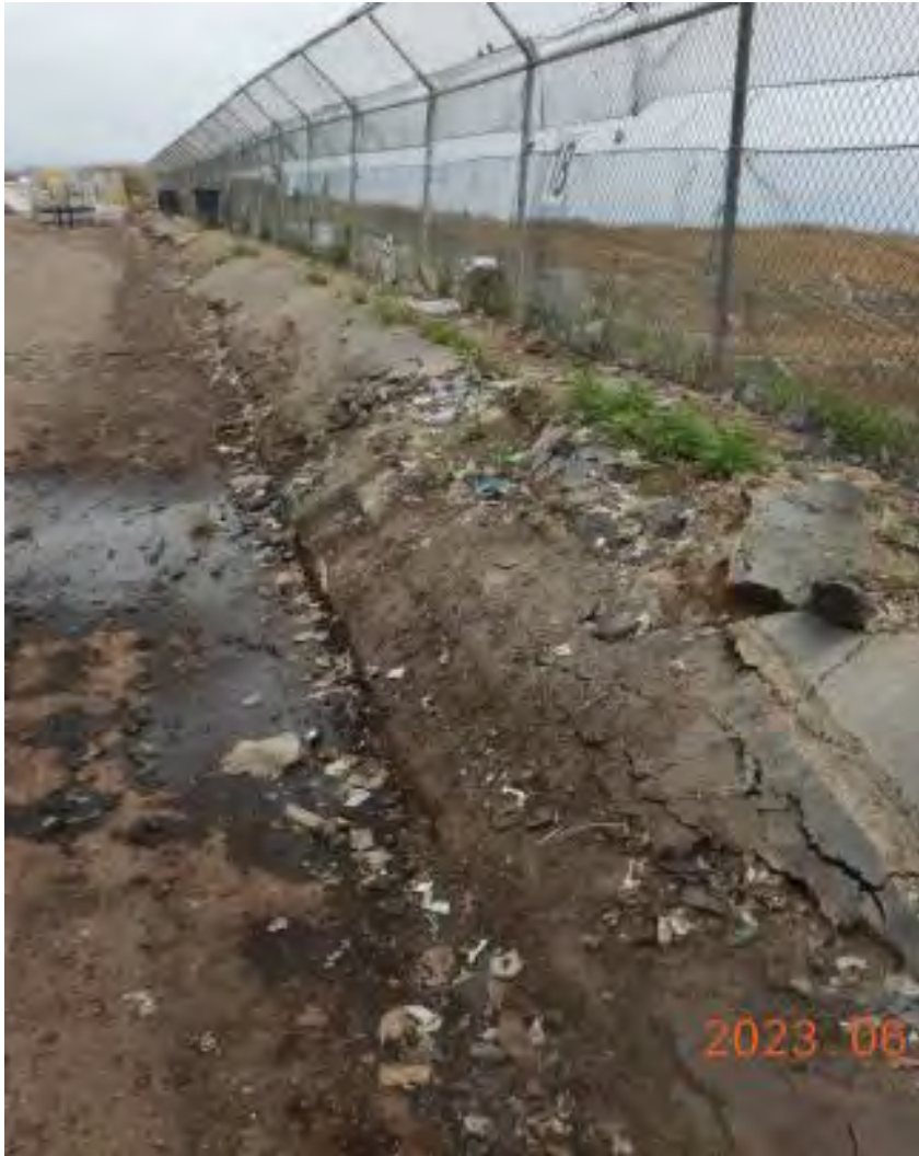
Photograph 19A. June 13, 2023. Damaged facility berm.
