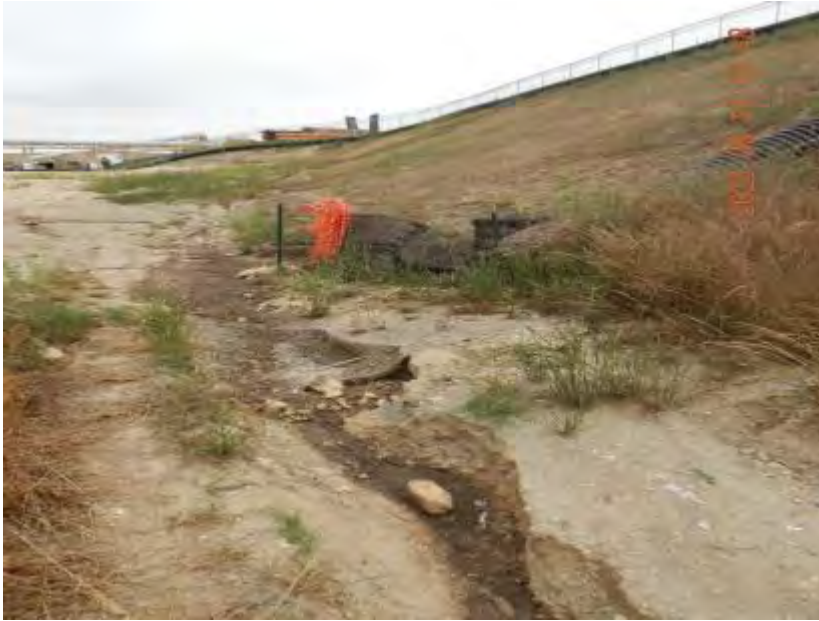
Photograph 37A. June 13, 2023. Wastewater flowing onto a landfill bench, over an unlined area of the landfill, where some wastewater enters a stormwater pipe while the remaining wastewater flows along bench into a second stormwater pipe. The first pipe (photo 32 and 33) connects to the north sediment basin and the second pipe (photo 34 and 37) connects to the south sediment basin.
