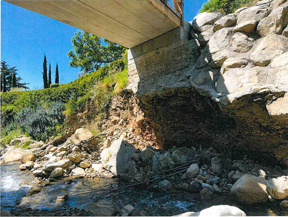
Figure 10 View of river right bank showing broken grouted RSP at bridge.
