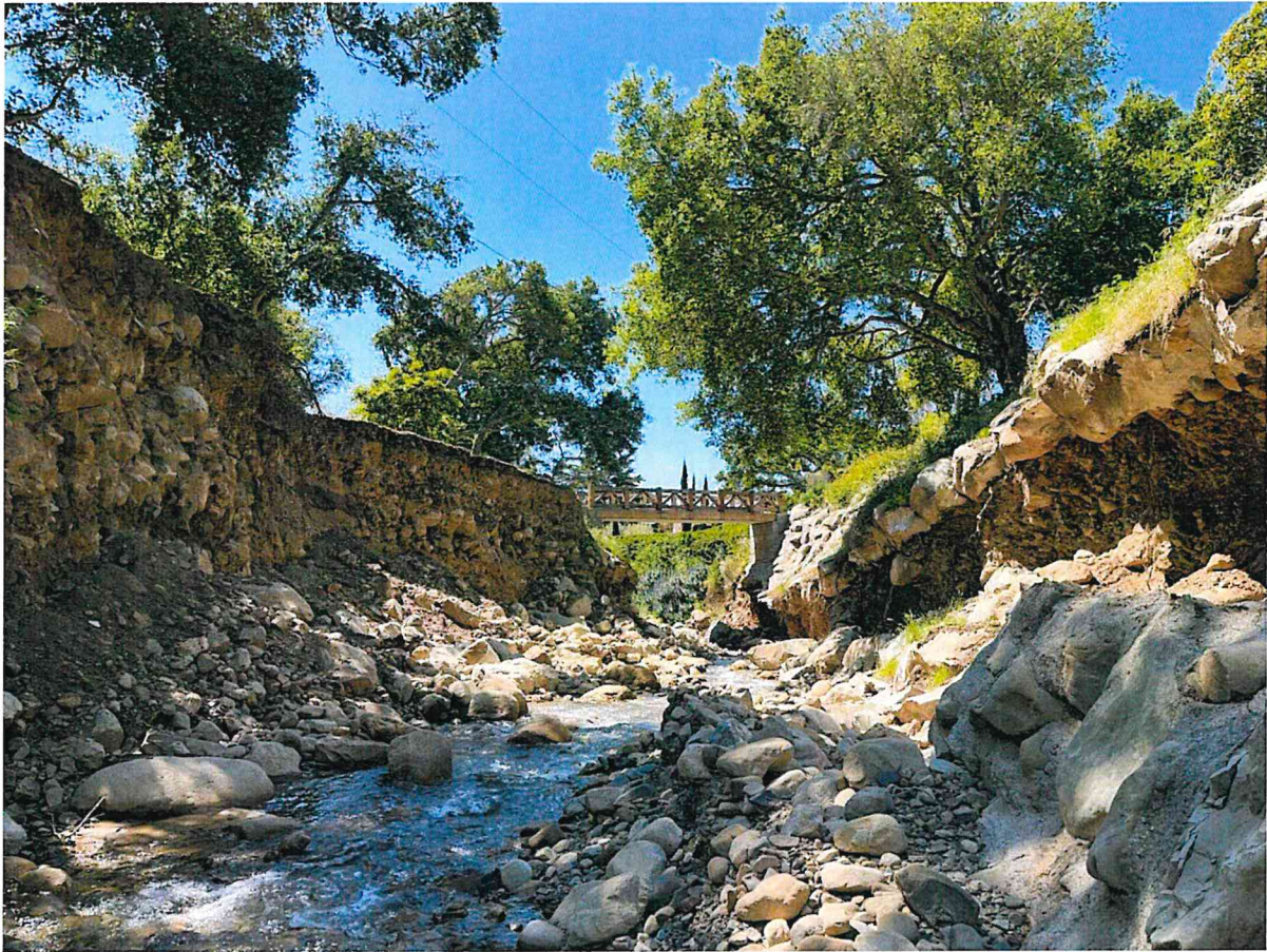
Figure 8 Looking downstream. Note incision and undercut RSP on river right.
