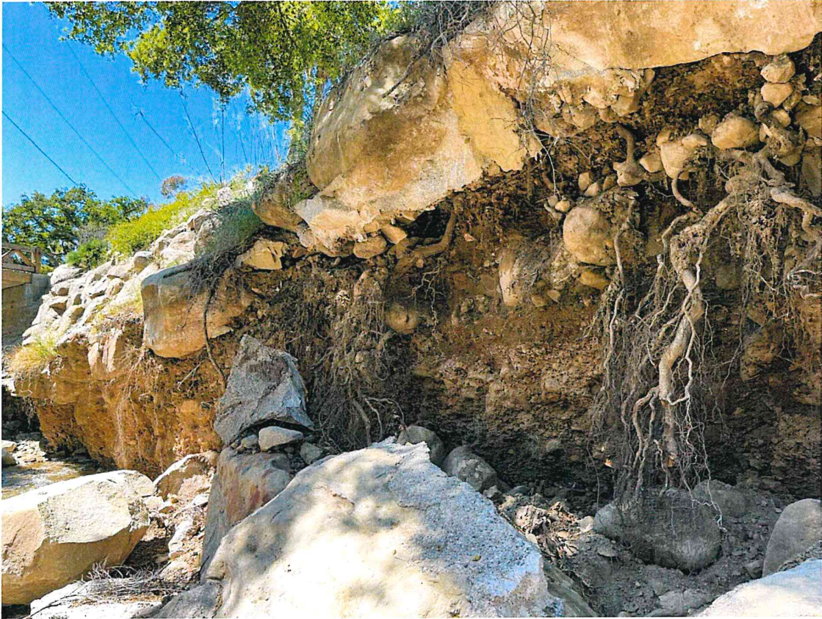
Figure 7View of ACOE grouted RSP upstream of new bridge on river right. Note concrete broken off where channel incised and now in stream channel.
