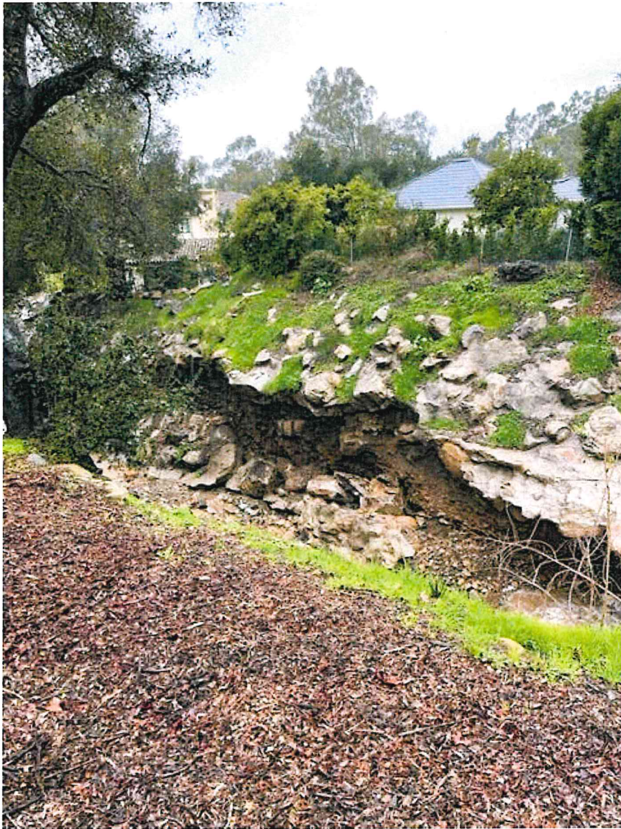
Figure 4 View of west bank of Romero Creek taken from east bank. Note the scour and broken sections of the grouted rock slope protection.
