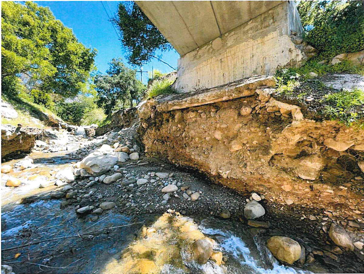
Figure 6 View of river left abutment looking upstream showing incision in creek. Note grade control structure upstream.
