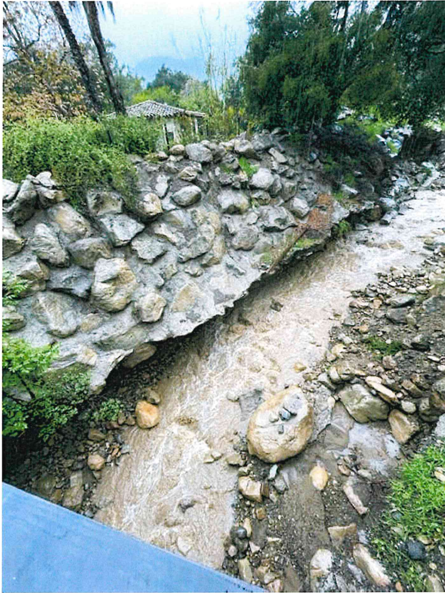
Figure 3 View of Romero creek looking upstream. Photo taken from bridge installed in 2022. Note undercut grouted rock slope protection.
