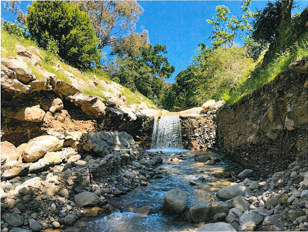
Figure 9ACOE installed grade control structure where channel further incised. note broken grouted RSP on left side of photo.
