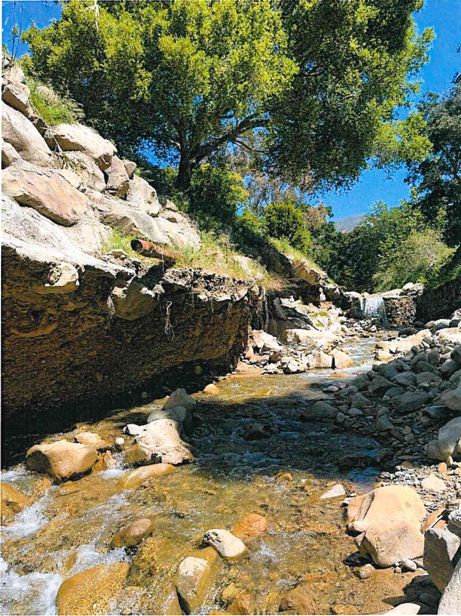
Figure 11 View of undercut bank between bridge and grade control structure on river right.
