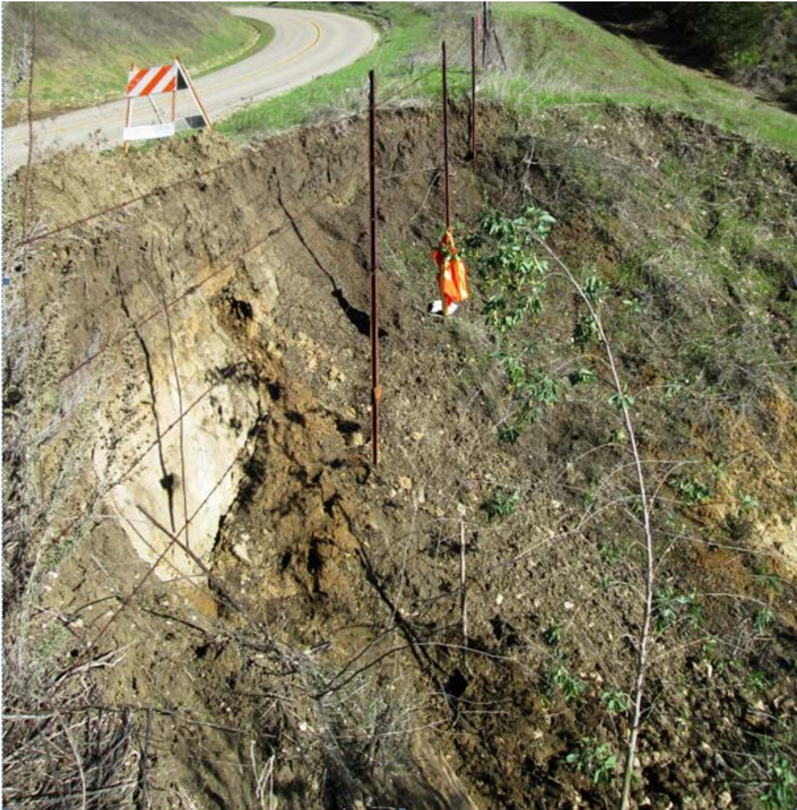
Figure 2-3 Bank Slip-out North of Bridge 17 on East Side of Road Looking North
