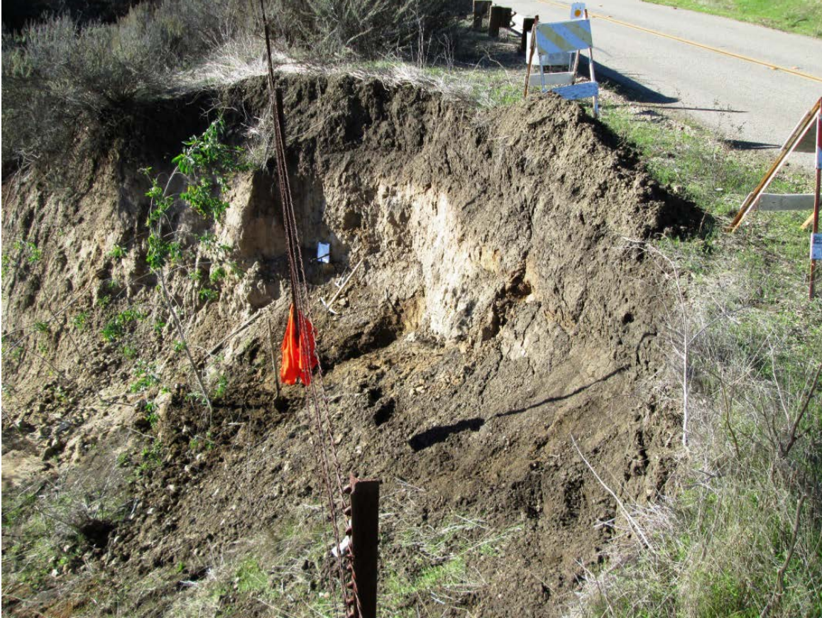
Figure 2-4 Bank Slip-out Area North of Bridge 17 on East Side of Road Looking SW
