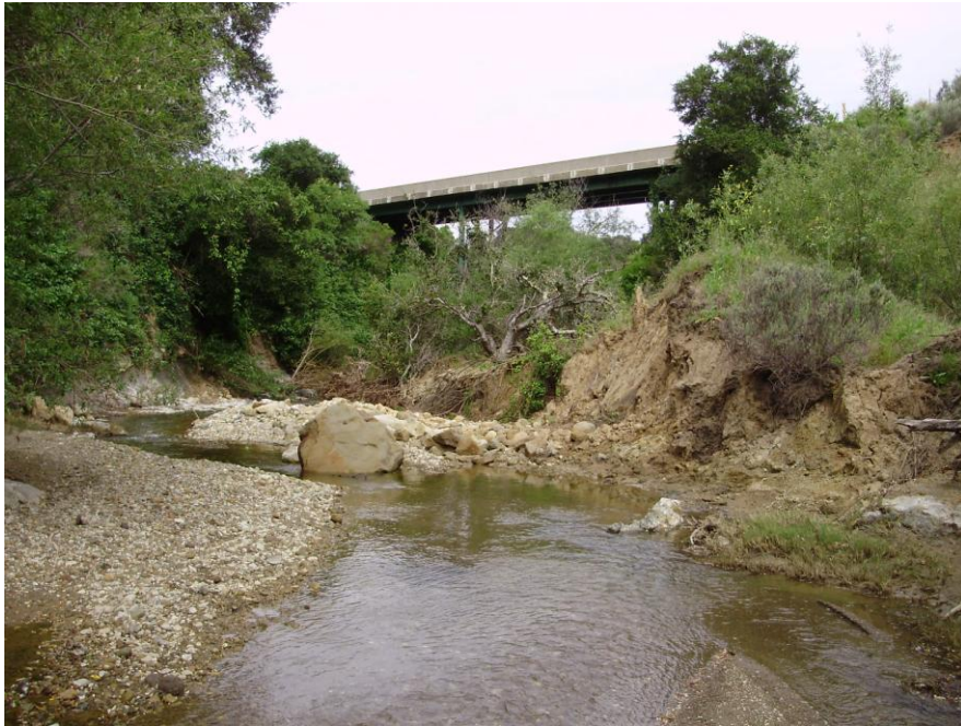
Photo 1. View of Jalama Creek from south of Bridge 17. Note the active bank slumping in the right of the photo.
