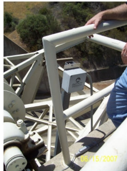
Dam Gate Inclinerometers
