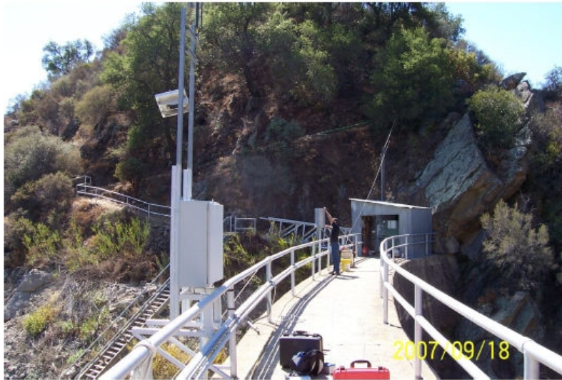
Reservoir Level & Rainfall ALERT Instrumentation
