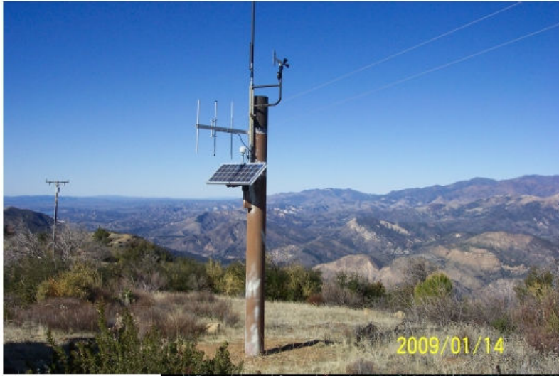
La Cumbre Peak Weather & Repeater Station
