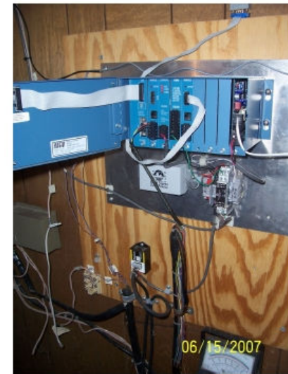
Reservoir Level & Gate Opening Data Interface to SB City (RUG9/SCADA)
