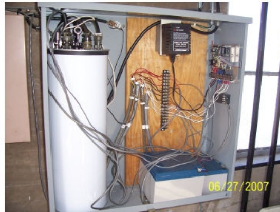
Reservoir Level & Gate Opening ALERT Instrumentation
