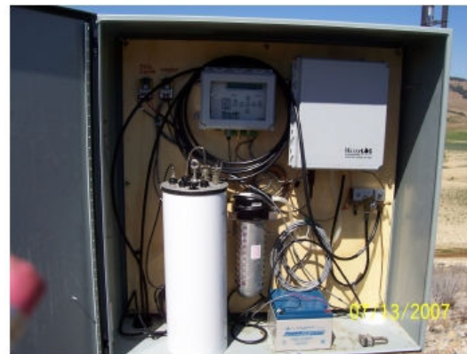
Reservoir Level ALERT Instrumentation (Bubbler)
