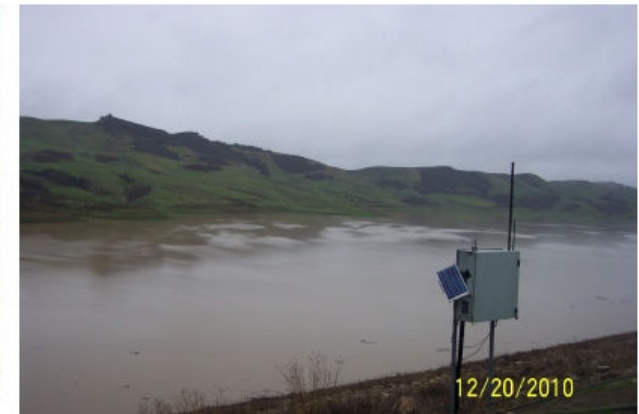
Twitchell Reservoir & ALERT Installation
