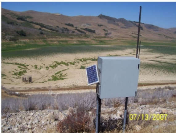
Reservoir Level Gauge Enclosure
