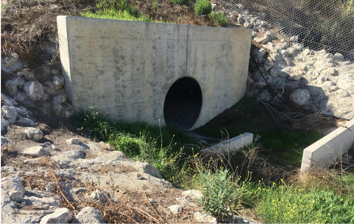
Photograph 5. Downstream terminus of below-ground pipe in western portion of study area draining into in-line detention basin and agriculture ditch, riprap feature visible on left. (aspect: south and upstream; November 1, 2018)
