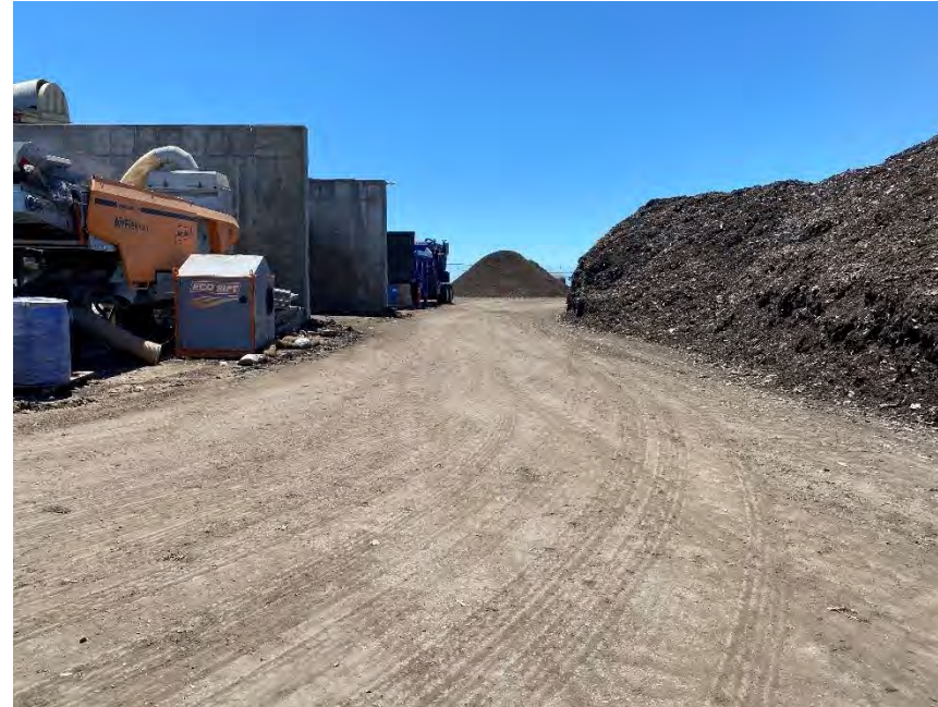
Photograph 22B. July 14, 2023. The working surface where feedstock/ digestate enters the facility from ADF has been repaired with asphalt.
