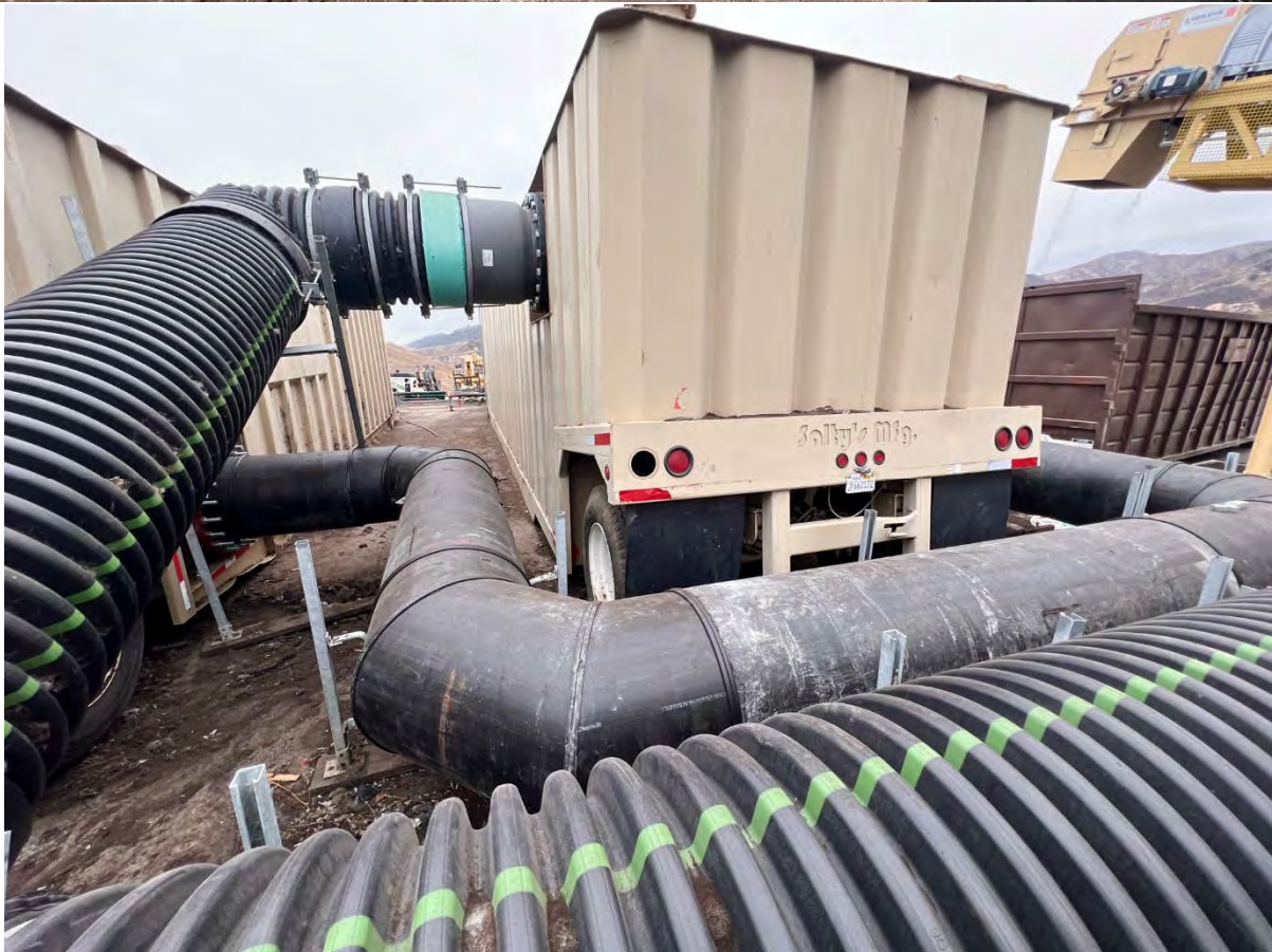
The conveyance system pipe repair is underway and currently scheduled to be completed prior to October 1, 2023.
