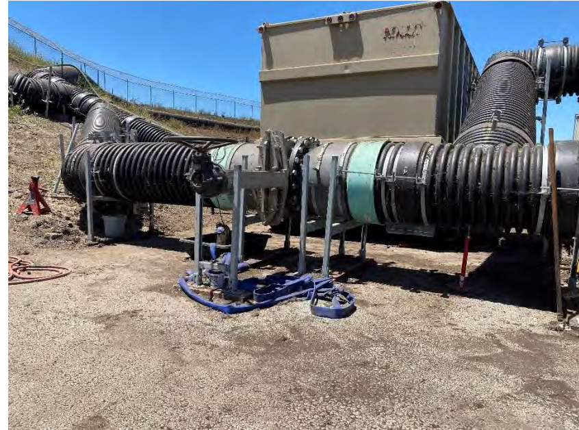
Photograph 28B. July 14, 2023. There is no longer collected wastewater below the conveyance system.
