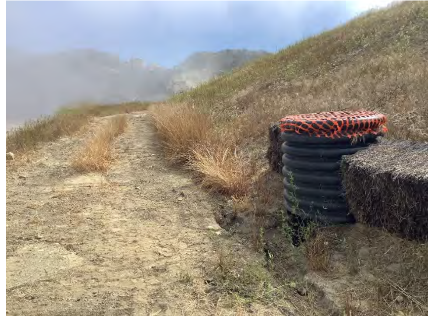
Photograph 34B. July 11, 2023. Stained soil has been removed and stored in a roll off bin.
