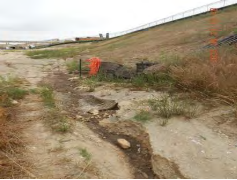
Photograph 37A. June 13, 2023. Wastewater flowing onto a landfill bench, over an unlined area of the landfill, where some wastewater enters a stormwater pipe while the remaining wastewater flows along bench into a second stormwater pipe. The first pipe (photo 32 and 33) connects to the north sediment basin and the second pipe (photo 34 and 37) connects to the south sediment basin.
