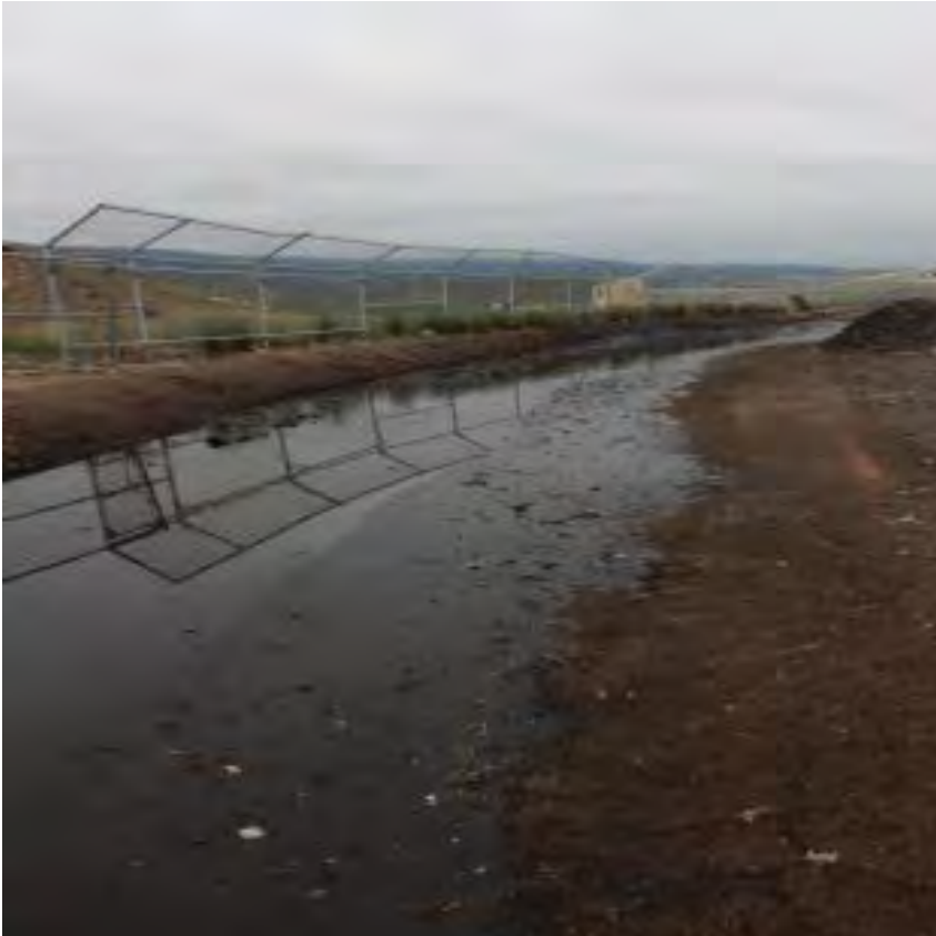
Photograph 8A. June 13, 2023. Pondered wastewater at the northern portion of the working surface.
