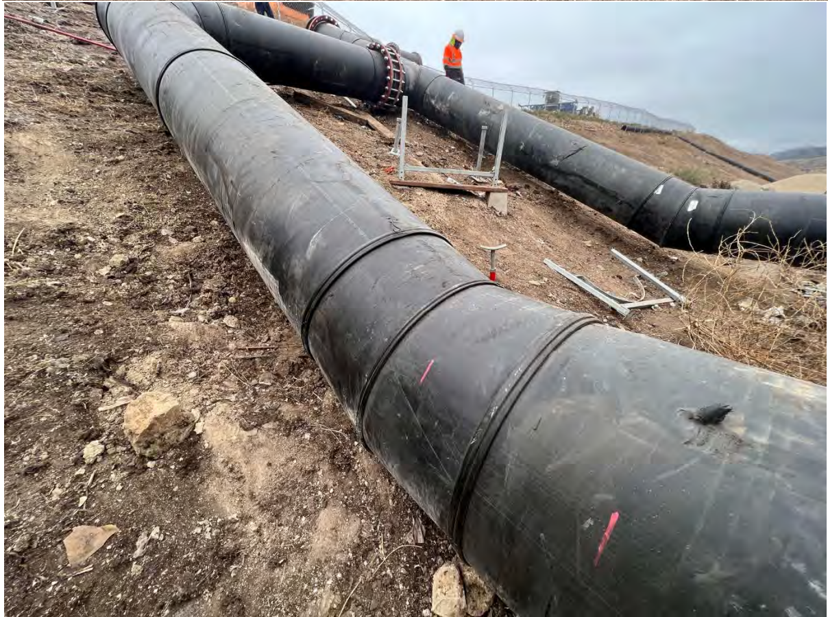
The conveyance system pipe repair is underway and currently scheduled to be completed prior to October 1, 2023.
