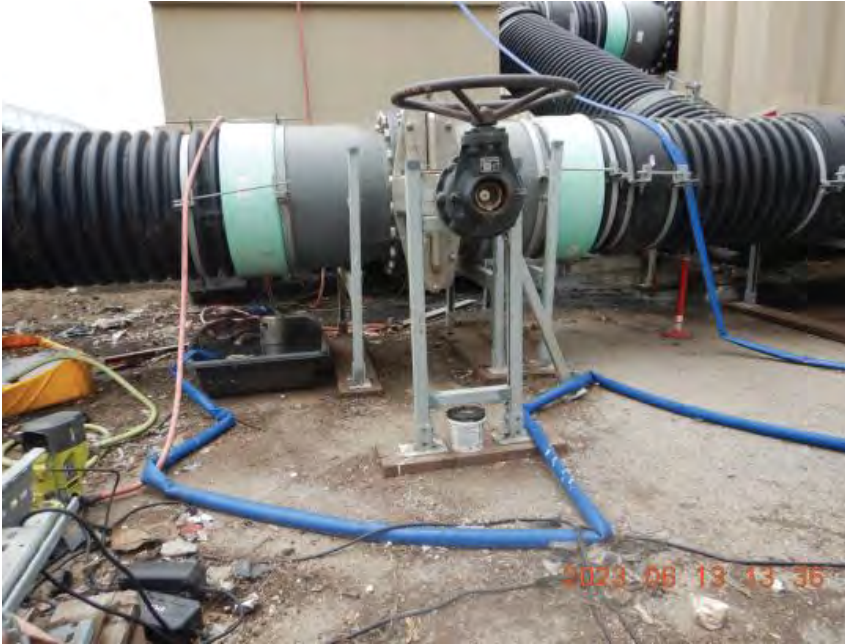
Photograph 30A. June 13, 2023. Wastewater actively flowing from damaged pipes.
