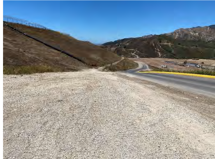
Photograph 26B. July 14, 2023. Stained soil has been removed and stored in a roll off bin.
