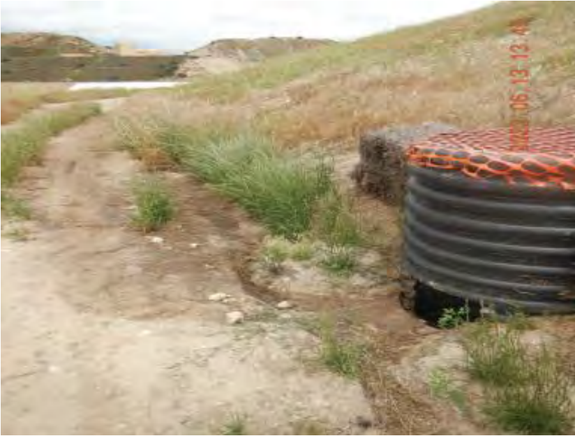
Photograph 34A. June 13, 2023. Wastewater flowing from the compost facility onto a landfill bench where it enters a second stormwater pipe connected to the south sediment basin.
