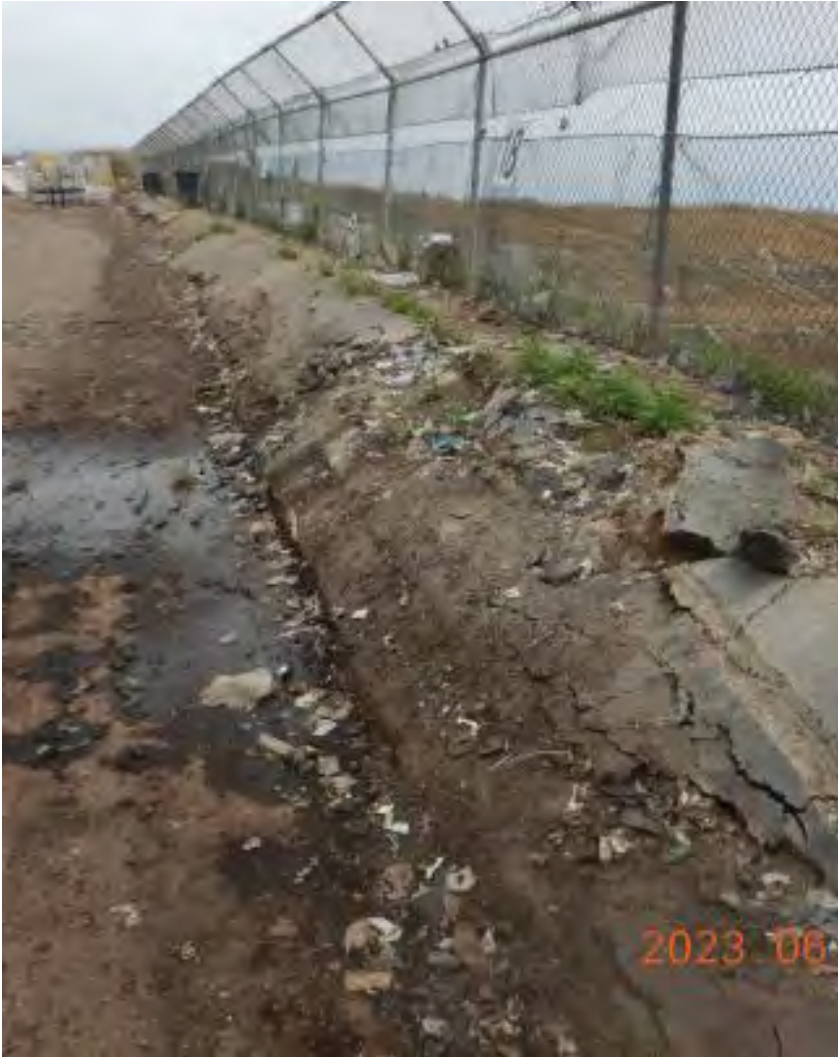
Photograph 19A. June 13, 2023. Damaged facility berm.
