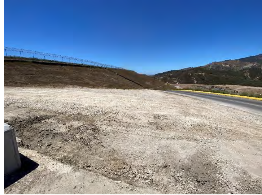
Photograph 25B. July 14, 2023. Stained soil has been removed and stored in a roll off bin.
