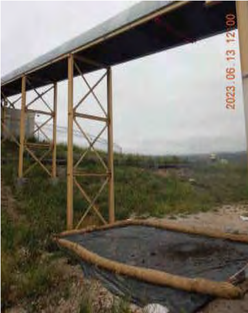
Photograph 1A. June 13, 2023. Conveyor system that moves compost feedstock (digestate) from the ADF to the CMU continues to have feedstock material beneath the conveyor from fallen material.
