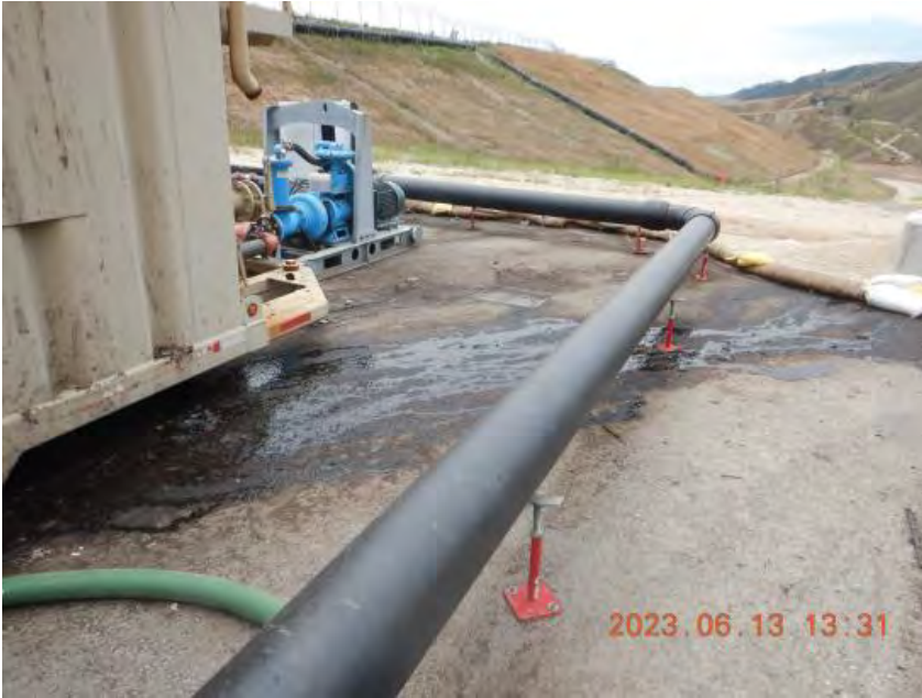
Photograph 23A. June 13, 2023. Wastewater flowing off D-table working surface.
