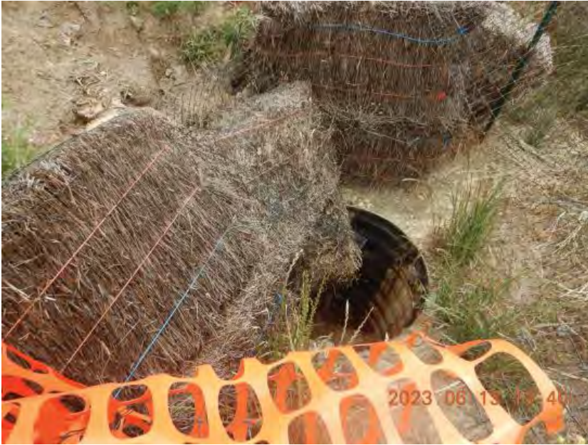
Photograph 32A. June 13, 2023. Pipe on bench where wastewater flows to the landfill north sediment basin.
