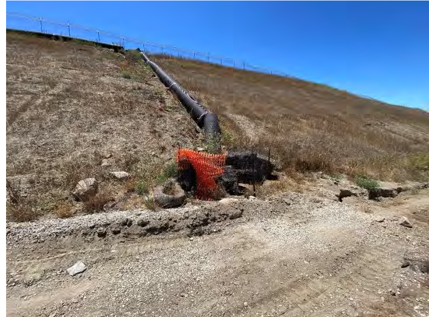
Photograph 32B. July 14, 2023. Stained soil has been removed and stored in a roll off bin.
