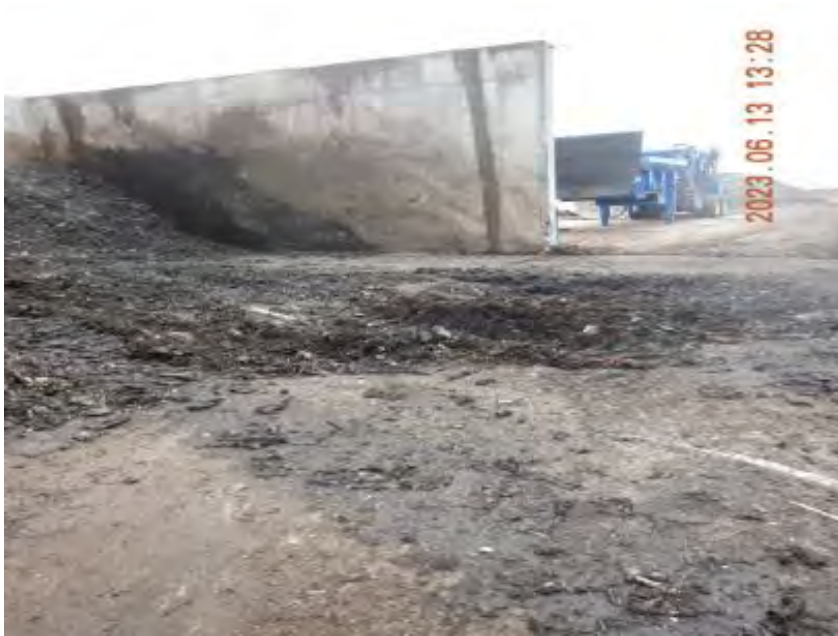
Photograph 22A. June 13, 2023. Damaged working surface where feedstock/digestate enters the facility from the ADF.
