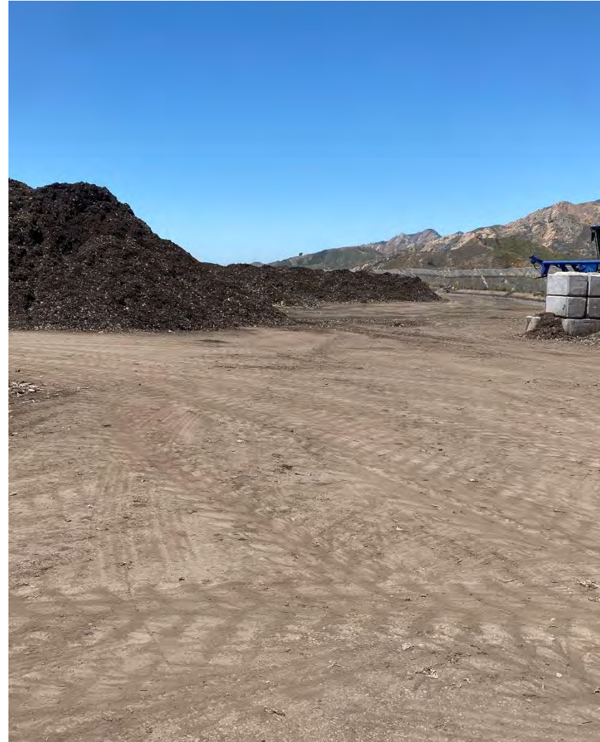
Photograph 11B. July 14, 2023. Damaged areas of the working surface have been repaired with asphalt.
