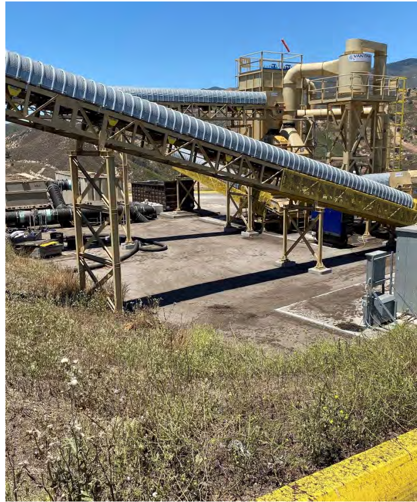
Photograph 2B. July 14, 2023. Asphalt berm has been installed to the west side of the baker tanks.
