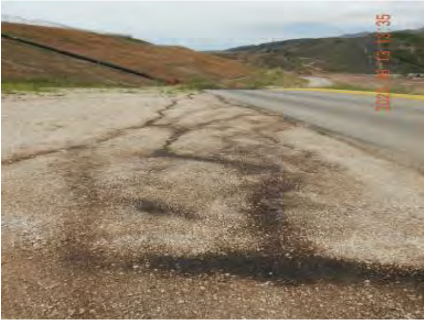
Photograph 26A. June 13, 2023. Wastewater flowing outside of the compost facility towards a lower landfill bench.
