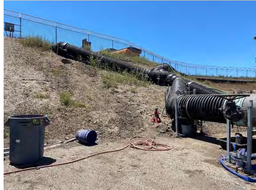
Photograph 27B. July 14, 2023. Stained soil has been removed and stored in a roll off bin.
