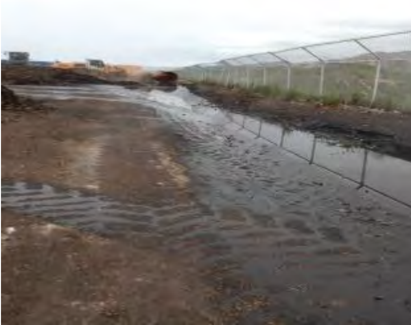
Photograph 9A. June 13, 2023. Pondered wastewater at the northern portion of the working surface with a scraper pushing compost/material into the ponded area after scraper dragged its blade around the perimeter of the working surface.
