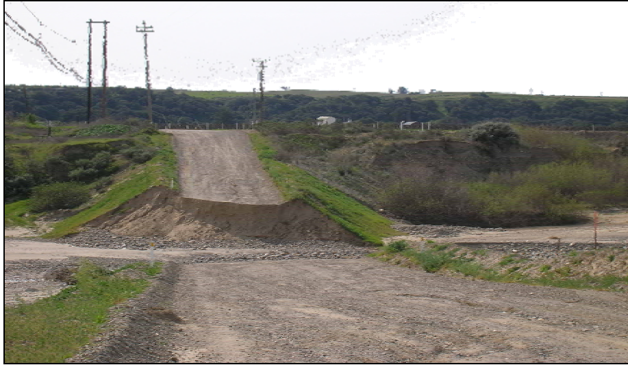
Photo: Existing Low-water crossing washed out.
