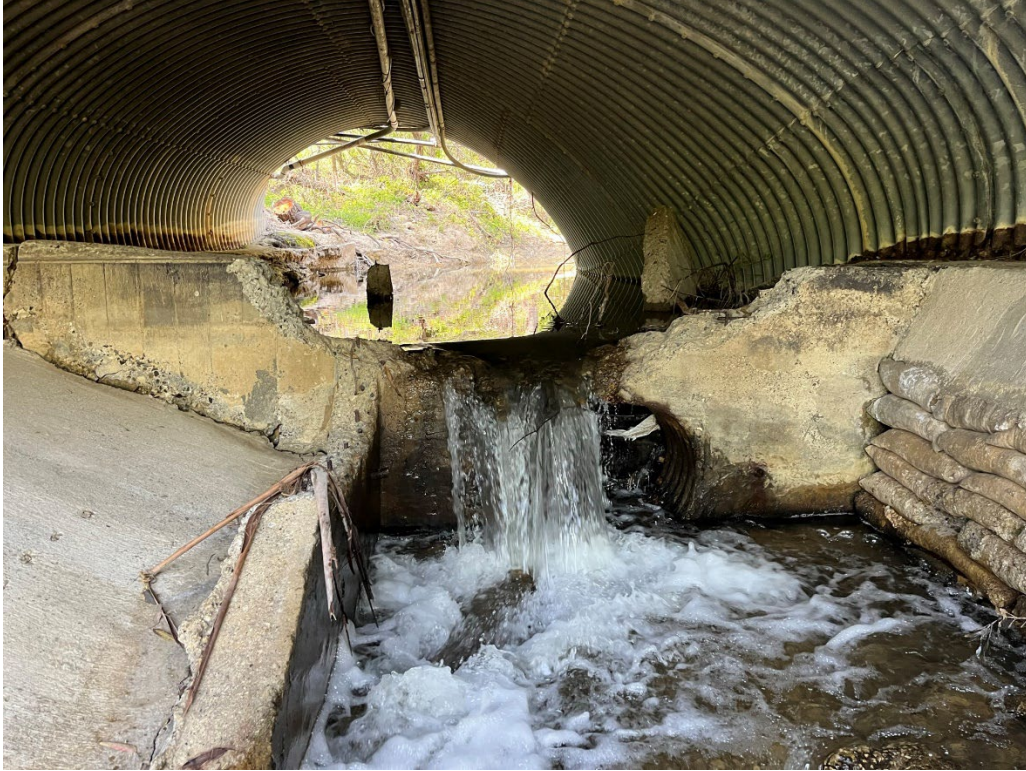
View looking upstream (north) at previous at grade concrete crossing and failed bottomless arch corrugated metal pipe culvert.
