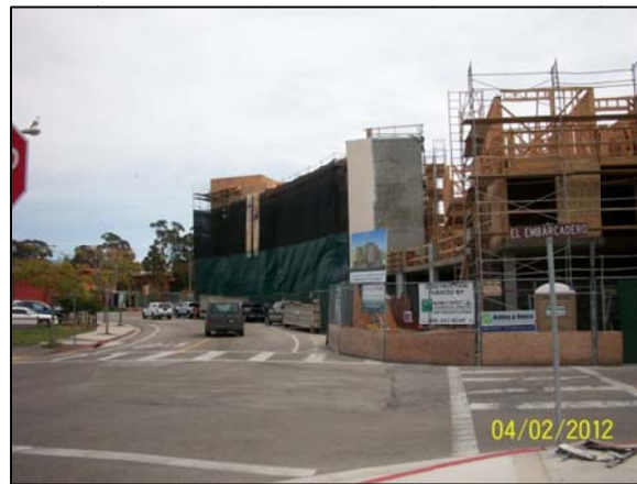
Infill, Remove and Reconstruct Concrete Sidewalk, Curb and Gutter and narrow roadway by 4-foot to allow for wider sidewalks, street trees (King Palm) and pedestrian scale street lights.
