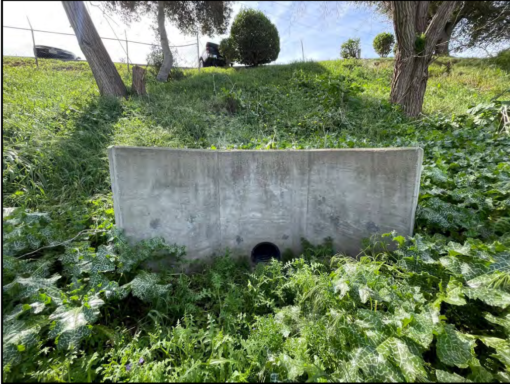
Photo 7: Culvert and headwall with surrounding ornamental trees and ruderal/disturbed understory in western portion of the Project Site (Aspect: South).
