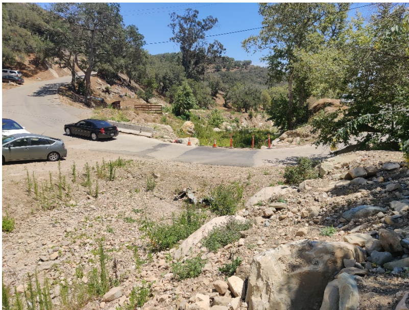
Existing Bella Vista low water crossing with plugged culverts
