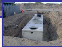
Jalama Beach Shower Leachfield System
