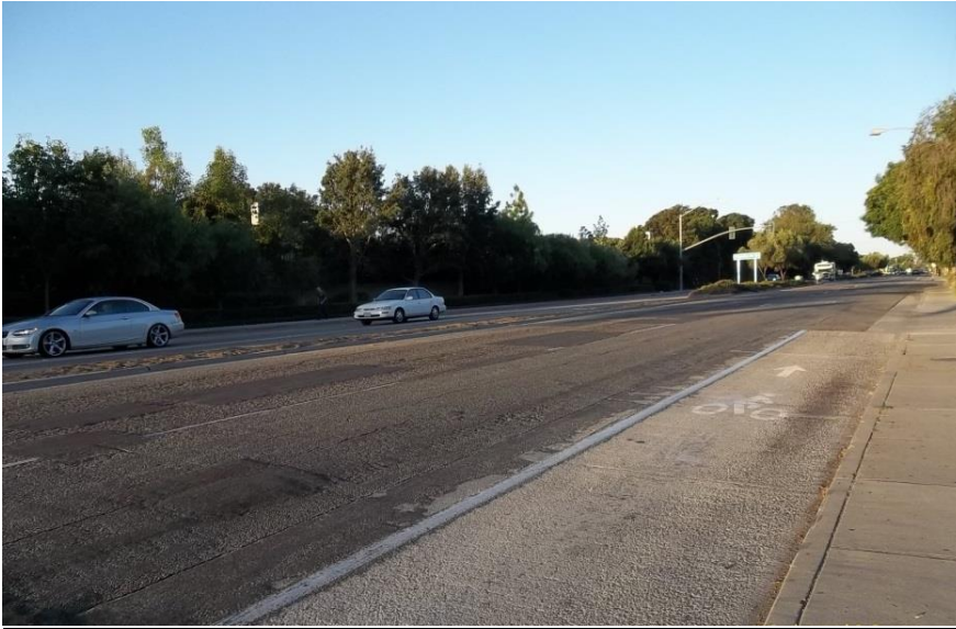
Typical damaged road bed that needs resurfacing on Hollister Avenue
