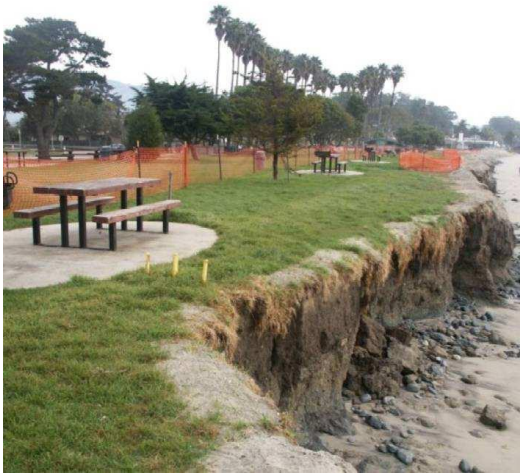
Family Picnic Tables and adjacent storm damage
