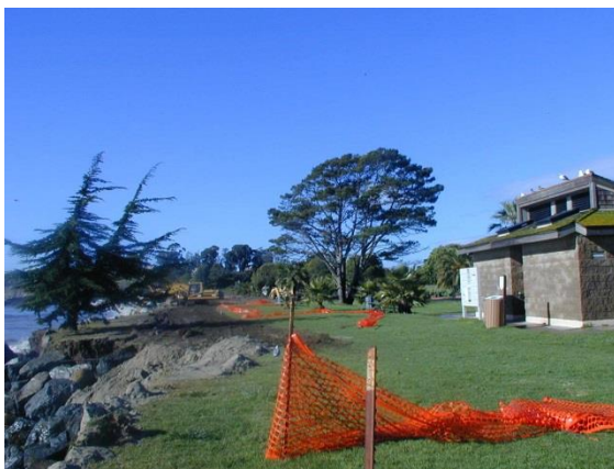
Park Erosion at existing restroom – 2002
