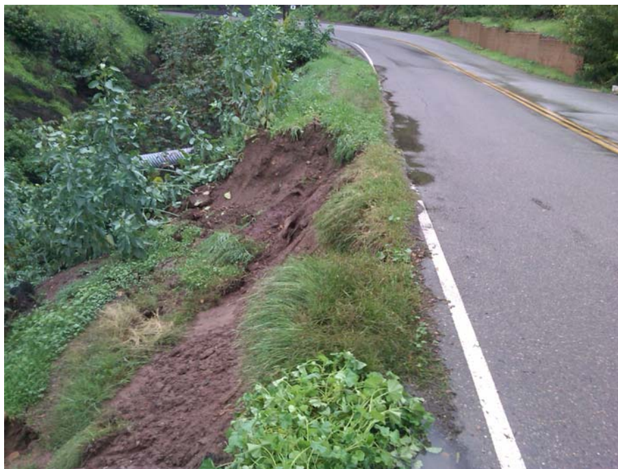
Reduced shoulder width at Tunnel Road MP 0.7(Site 1A02)
