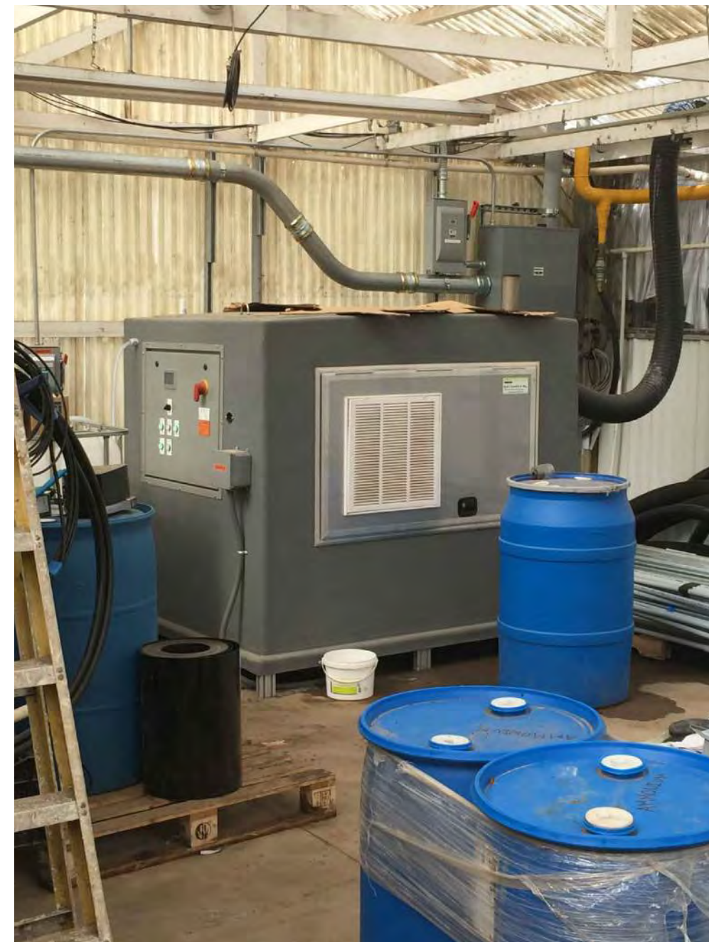
ODOR CONTROL UNIT
