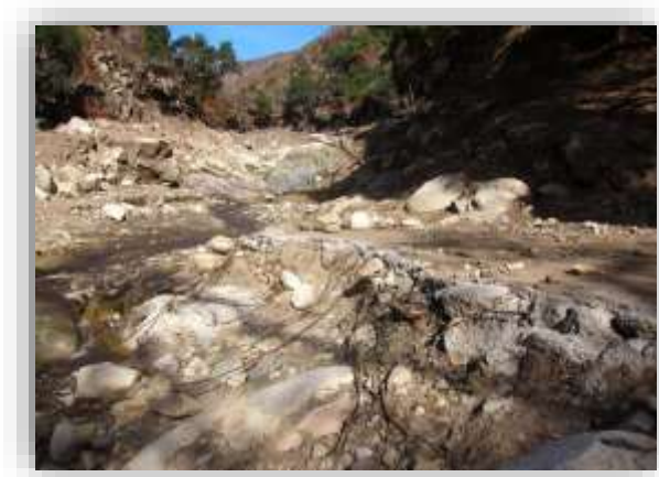
Low Water Crossing Post-Thomas Fire Debris Flow Incident, January 2018 (view west)
