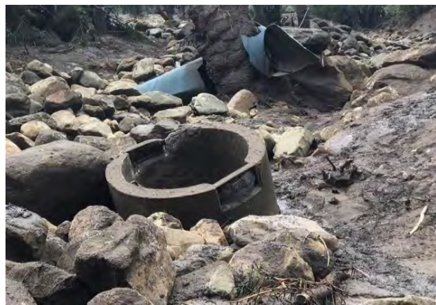
Damage to SCC vault after 1/9/18 debris flows
