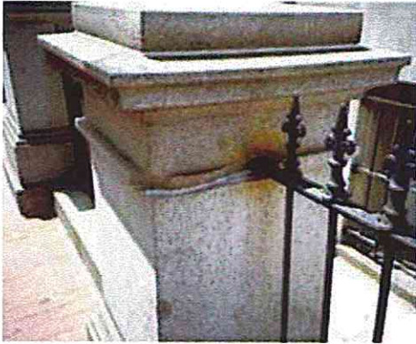
The iron stain on this granite post may be removed by applying a commercial rust-removal product in a poultice. Photo: NPS files.
