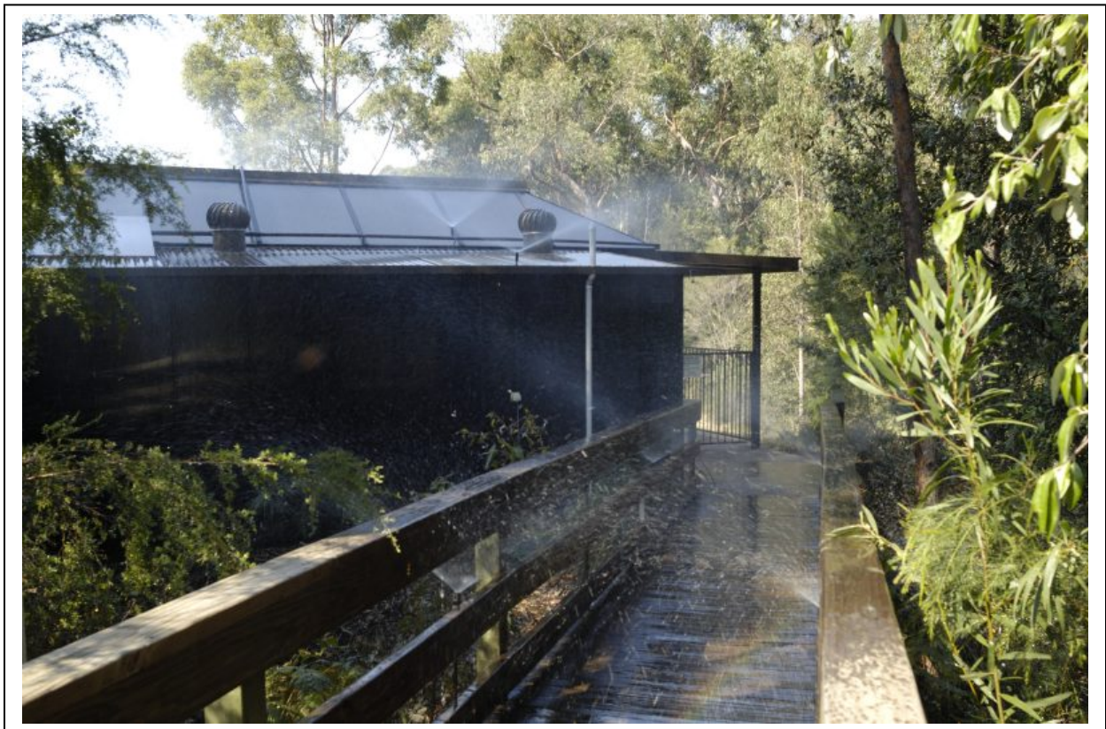
Figure 6. External sprinklers. As a wildfire approaches, external sprinklers wet the structure at risk, the surrounding environment, and increase the local humidity to prevent ignition. Photo: A conference center in New South Wales, Australia.
