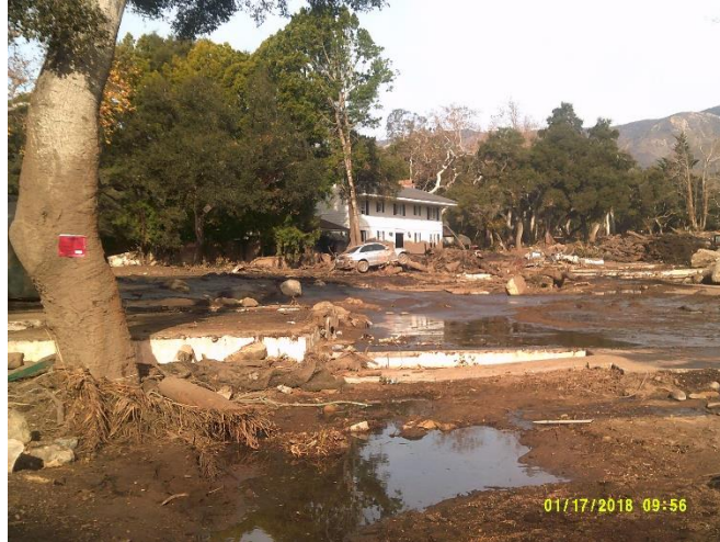
Hot Springs Road. Debris flow entered roadway and shoulder, damaging and destroying AC dike, drainage inlets, and traffic control signs. Debris flow, heavy excavation and hauling operations damaged the pavements marking, striping and roadway surface.
